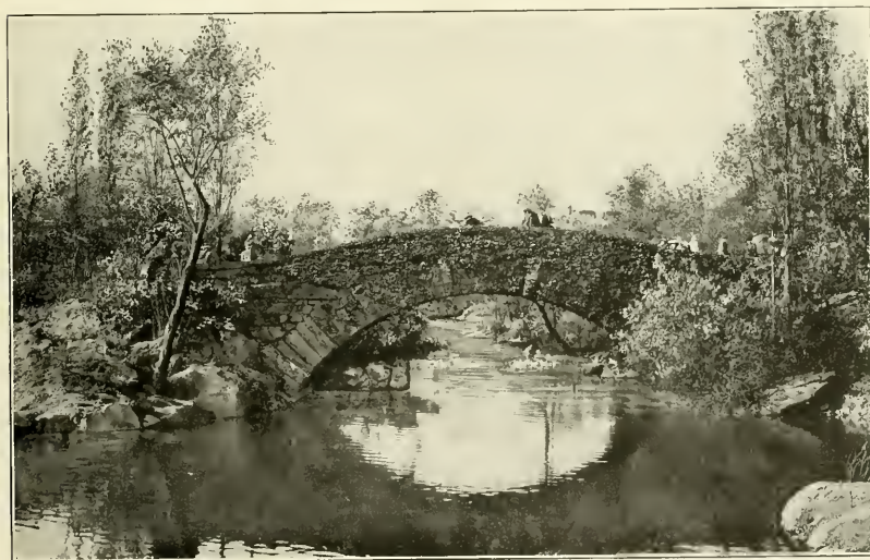
VINE ARCH BRIDGE —Central Park extends between Fifth and Eighth Avenues from 59th to 110th Street, being one of the largest and most beautiful parks in the world. The Vine Arch Bridge is one of the most picturesque sights and is a very popular spot for all lovers of nature.
