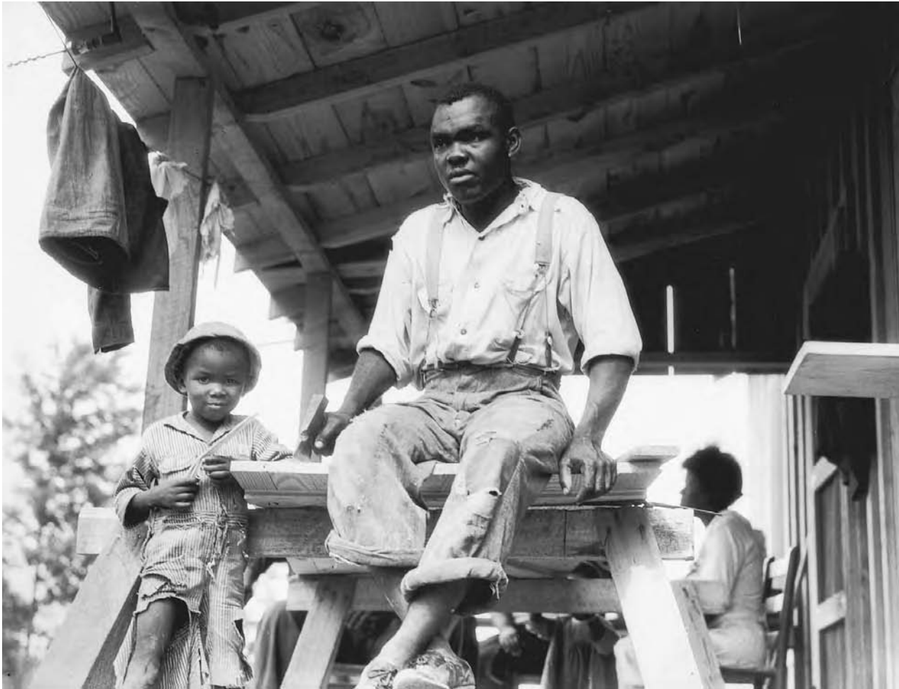
An evicted Arkansas sharecropper, an active member of the Southern Tenant Farmers Union, builds a new home near Hill House, Mississippi, in 1936. LIBRARY OF CONGRESS, PRINTS & PHOTOGRAPHS DIVISION, FSA/OWI COLLECTION
