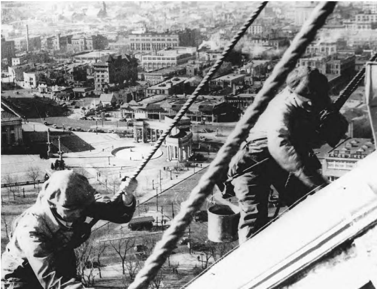
Men employed by the Civil Works Administration clean and paint the dome of the Denver capitol building in 1934. NATIONAL ARCHIVES AND RECORDS ADMINISTRATION
