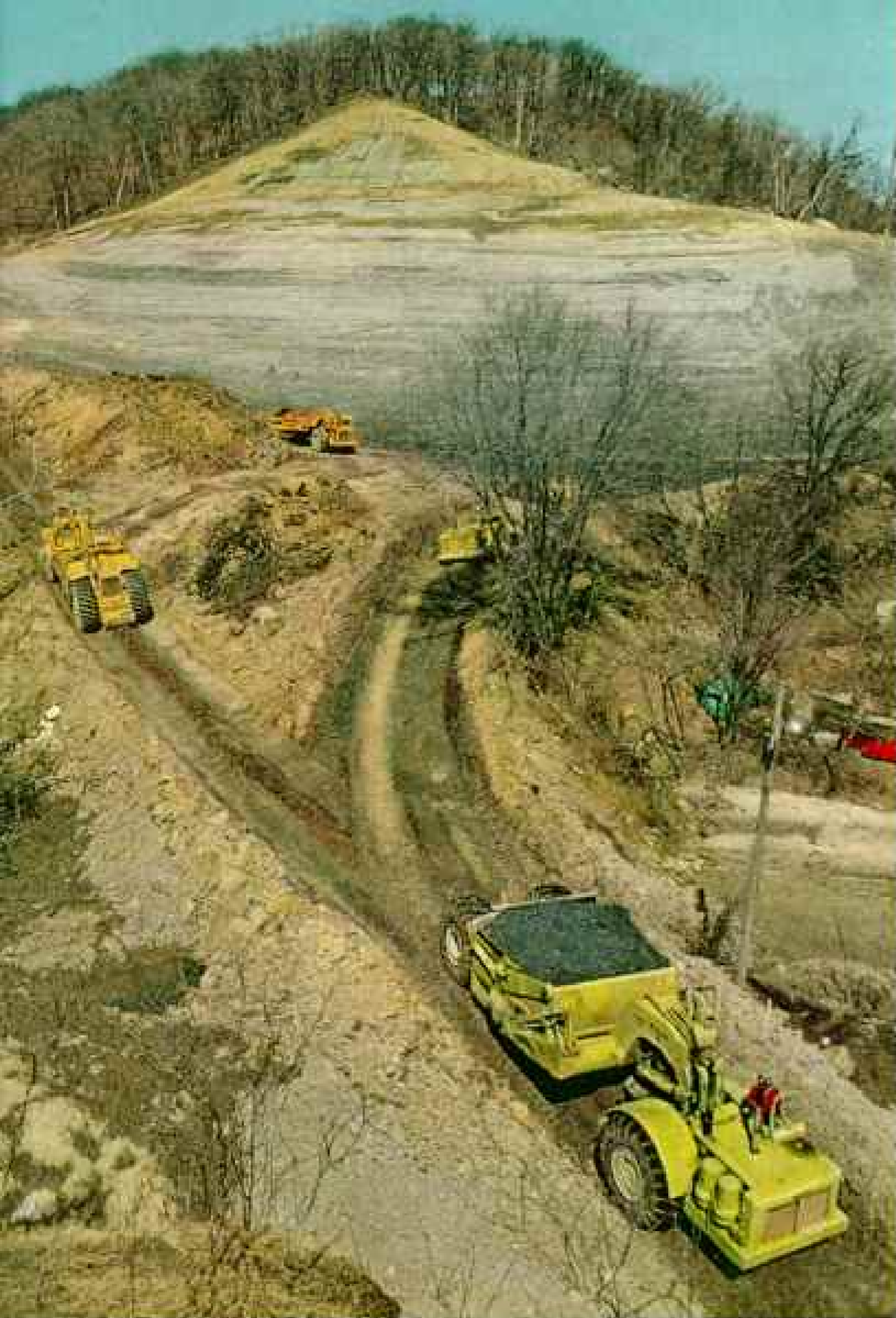
Moving a hillside to tame a river: Hungry scrapers gulp huge loads of earth to build up a North Mankato dike. The region's rich blue-gray clay proved ideal for making watertight levees.
