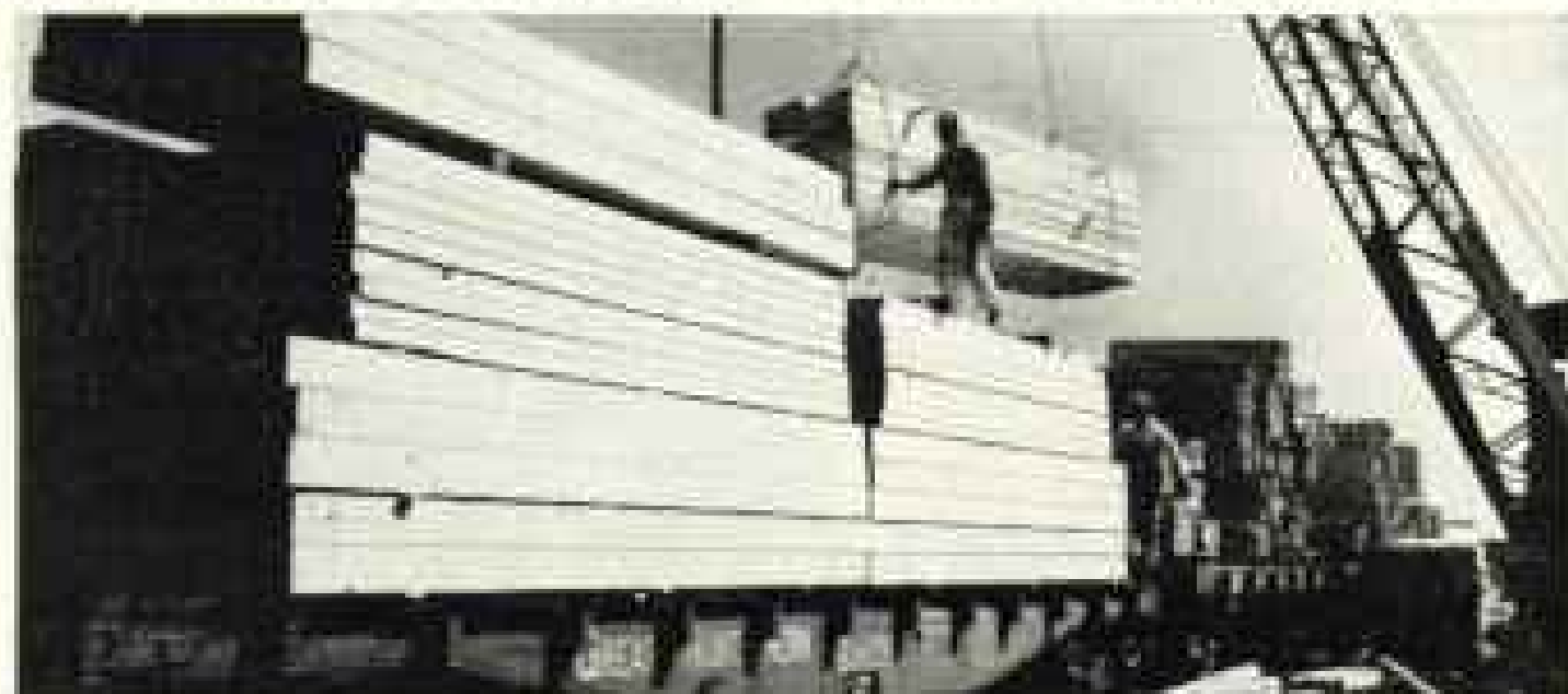
The dependable handling of lumber and other timber products is one of the many things that make Great Northern great.
