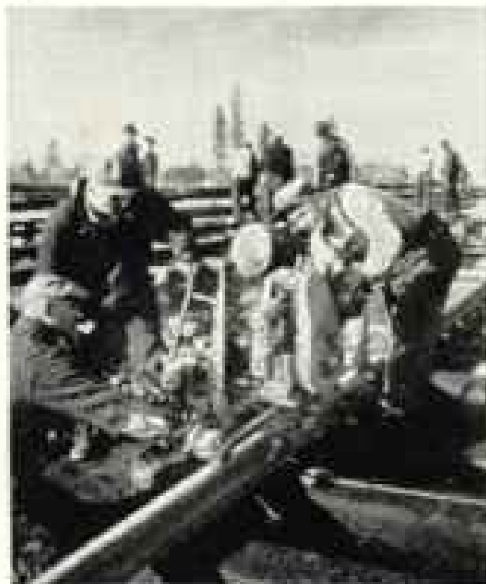
Installing new track. The machine drills holes thru the steel so that rail ends can be bolted solidly together.
