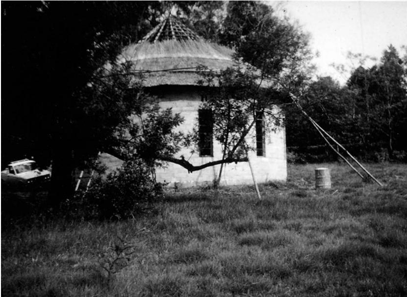
Plate 6.2 USPG mission church under construction at Mankaiana, western Swaziland, 1969. The first Anglican church in Swaziland was built of brick in 1881 and would not have looked out of place in a British town; it was subsequently abandoned. Out-station churches were later built in a more vernacular style, with thatched roof and cow-dung floor.
