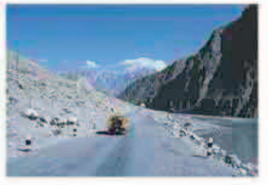
▲ The Karakoram Highway linking Mansehra in northern Pakistan with Kashi in western China was finally completed in 1978, 20 years after construction began. Regular mudslides and rockfalls necessitate continual maintenance for the road to remain open.
