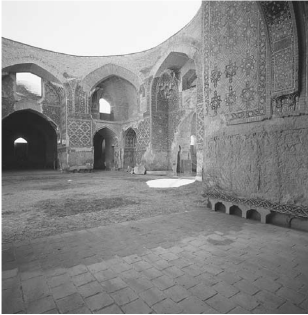
The ruins of the Blue Mosque in Tabriz, built in 1465 and later damaged by an earthquake. (ROGER WOOD/CORBIS)
