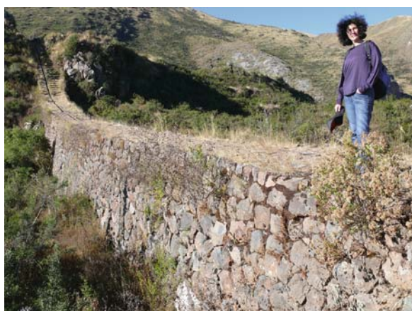
Fig. 9.18 Elevated portion of main aqueduct in Tippon (photo copyright by Yuri Gorokhovich)
