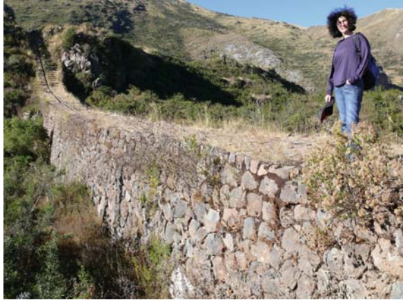
Fig. 9.18 Elevated portion of the main aqueduct in Tipon (photo copyright by Yuri Gorokhovich). Color version available in Appendix
