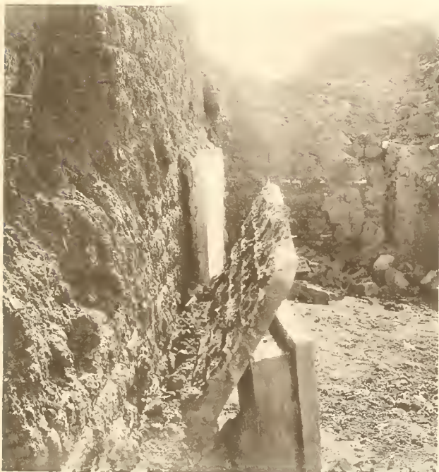
STONE LINING PARTLY FALLEN FORWARD.
