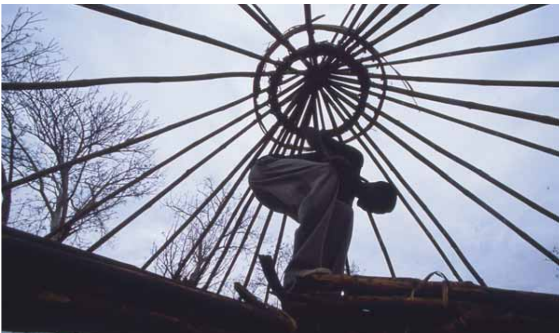
Refugees who fled violence in Fugnido camp (Ethiopia) construct new shelters in Bonga camp, Ethiopia, 2003.
