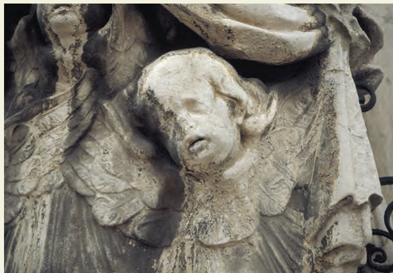
▲ Buildings Acid rain has eroded and eaten away the face of this stone angel in London, England (National Geographic Image Collection).
