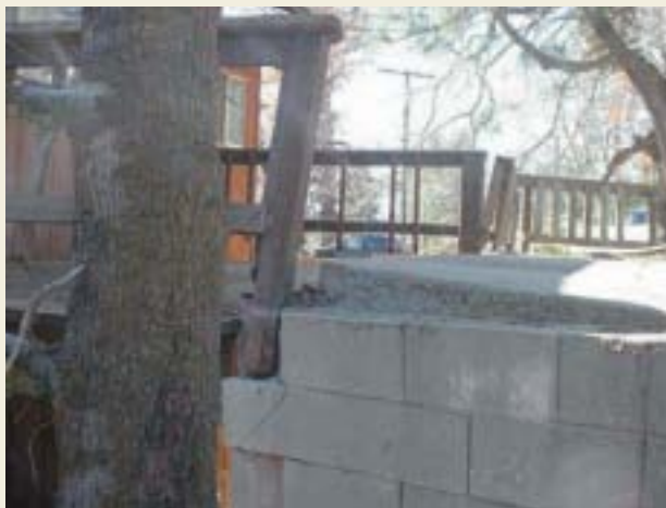
The concrete driveway slab here has been heaved upward by expansive soils, also causing damage to the adjacent railing and retaining wall.
