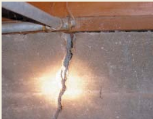
Foundation cracks like this one, caused by expansive soils, can cause serious damage to buildings that is expensive to repair.
