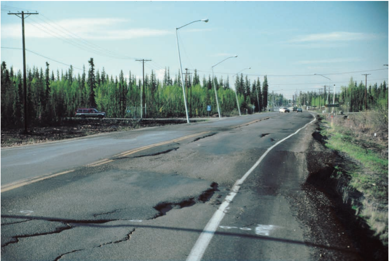
Figure 19.2 Road subsidence passing between leaning light poles in Alaska as a result of frost heave. (Source: Larry D. Hinzman, University of Alaska Fairbanks)
