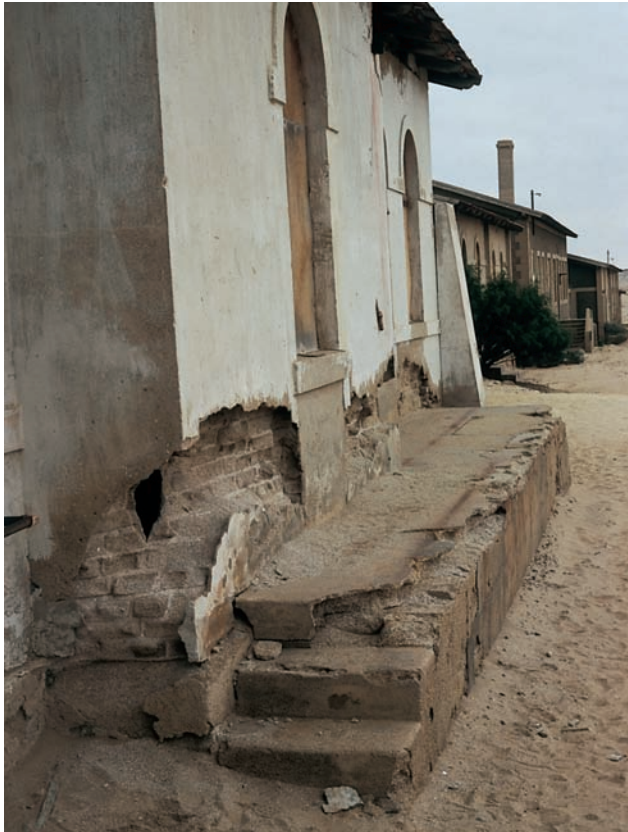
Figure 16.27 Wind erosion of a building. The height of the erosion notch represents the height of grain saltation, Kolman-skop, Namibia.
