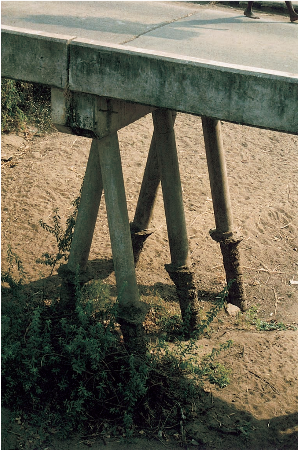
Figure 14.20 Exposure of bridge piers on a tributary of the Luangwa River, Zambia. The original bed level can be seen by the 'ragged' concrete on the piers.
