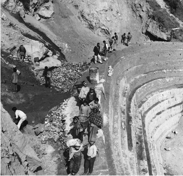
Figure 6.8 Darjeeling Highway, West Bengal, India. In October 1968 the Darjeeling Himalaya experienced a rainstorm of over 1,000 mm in a three-day period. Thousands of landslides were released and the 50-kilometre highway between Siliguri on the Terai and Darjeeling was cut in 52 places. Here one of the major landslide breaks is undergoing massive and expensive repair, November 1968.
