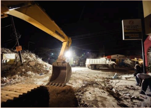
Figure 13.5 Cleanup efforts in Haiti after the 2010 earthquake
