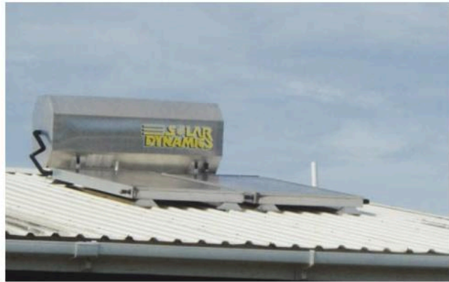
Figure 7.38 Solar heater to provide hot water in Barbados
