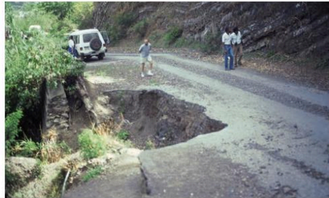
Figure 2.1 Road collapse in the Blue Mountains, Jamaica
