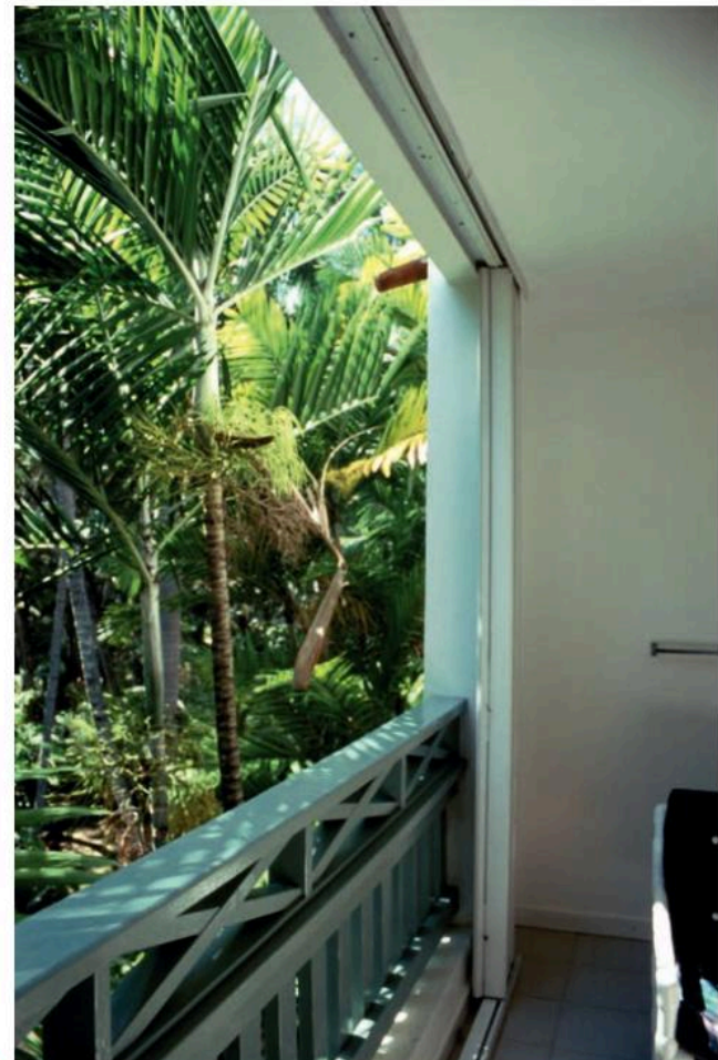
Figure 13.23 Storm shutters to protect against a hurricane
