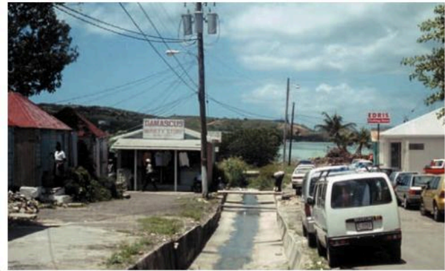
Figure 13.28 Paved drain in St John, Antigua
