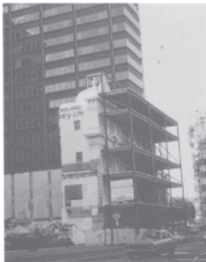
Fig. 3.1 (left) Facadism: the front of an old building is propped up before a modern addition is built behind it in Brisbane, Australia.
