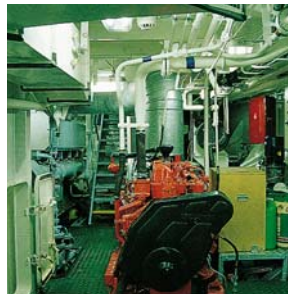
la sala macchine engine room
