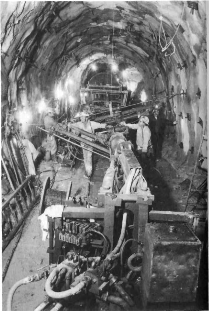
ILLUSTRATION 14 - Miners at work in tunnels beneath Rainier Mesa at the Nevada Test Site. They're stabilizing the walls with rock bolts and epoxy so that when the nuclear explosions go off, the walls won't crumble. Department of Energy photo.
