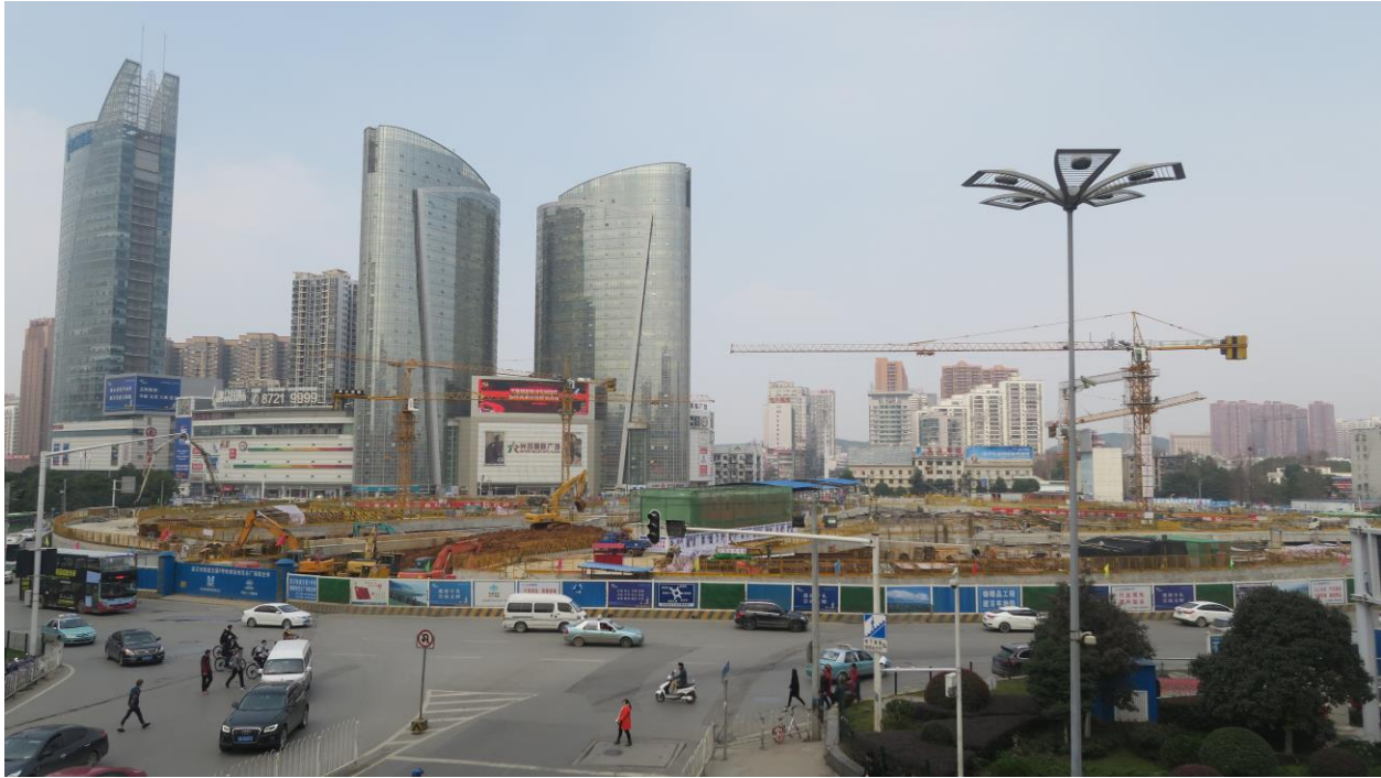
Figure 1 Ongoing construction at Optics Valley roundabout, the gateway to Wuhan's East Lake Hi-Tech Development Zone (Photo: Robert Cowley)
