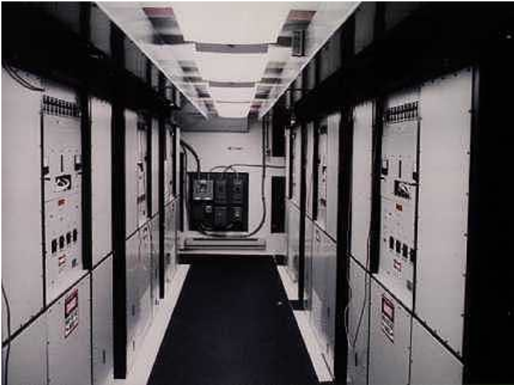
Image 4: Inside the Transmitter Shelter
