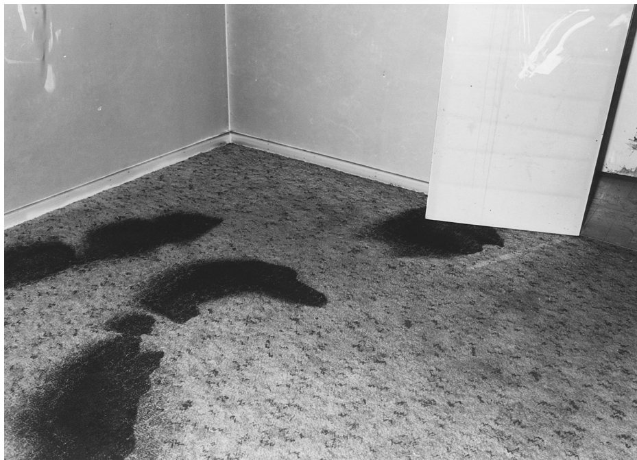
Figure 15.2 Burn patterns in carpet is the most valuable indicator of the involvement of flammable liquids in fires. However, there are several other potential causes for these patterns including, burning materials falling to the floor, 'shadowing' by items on the floor and burning characteristics of some types of carpet materials. In this example, all alternatives other than the presence of a flammable liquid were eliminated, and the sample was subsequently found to contain petrol
