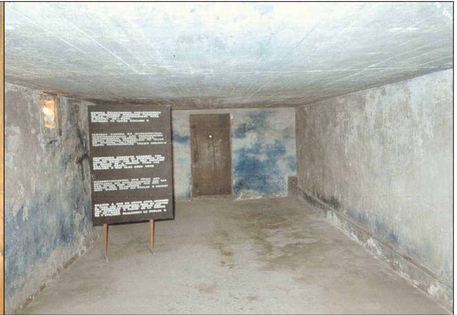
Color Illustration 7: Blue staining on the walls of chamber III of the delousing facility in hut 41 (“Bad und Desinfektion I”), concentration camp Majdanek. © C. Mattogno
