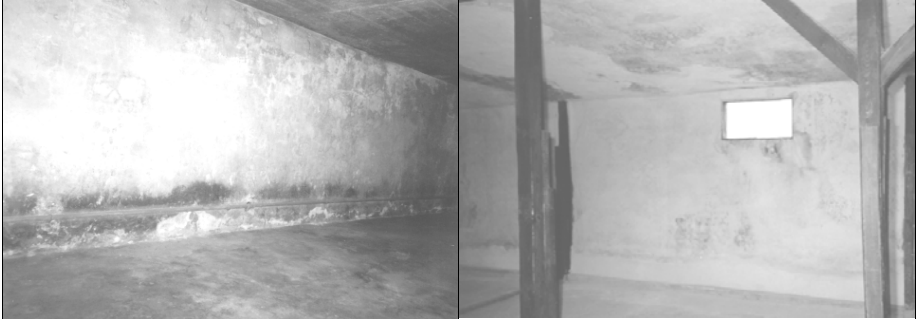
Illustration 7: Blue staining around the pipe near the floor of the eastern wall of chamber III of the delousing facility in hut 41, concentration camp Majdanek (cf. color picture on back cover; cf. map, illustration 1). © C. Mattogno
