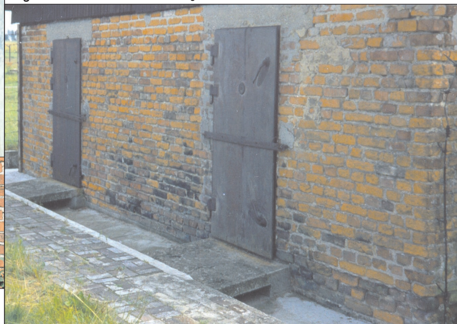
Color Illustration 5: Blue staining on the exterior walls of the delousing facility in hut 41 (Bad und Desinfektion I), concentration camp Majdanek. © C. Mattogno
