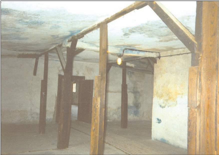
Color Illustration 6: Blue staining on the walls and ceiling of chamber IV, hut 41, (delousing gas chamber in “Bad und Desinfektion 1”), concentration camp Majdanek. © C. Mattogno
