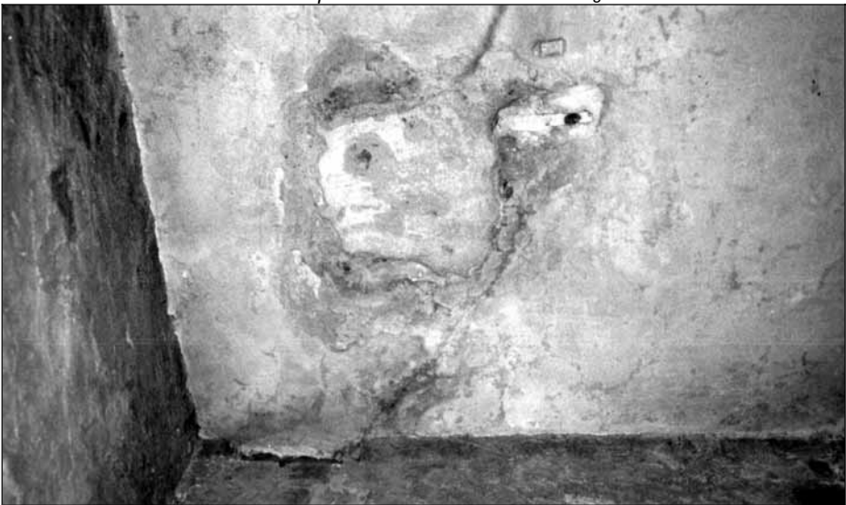
Document 19: Photo of opening no. 1 in the roof of the vestibule, part of the former morgue. © Carlo Mattogno
