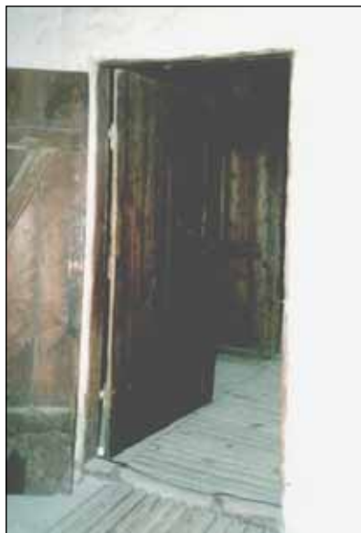
Photograph XVII: Barrack 41, gas chamber, north door. The inside of the door is marked by the typical discolorations that are also visible on the outside of the south door (Photograph XVIa); hooks for the latches are missing from the door frame, unlike on the frame of the south door (Photograph XVI). © Carlo Mattogno
