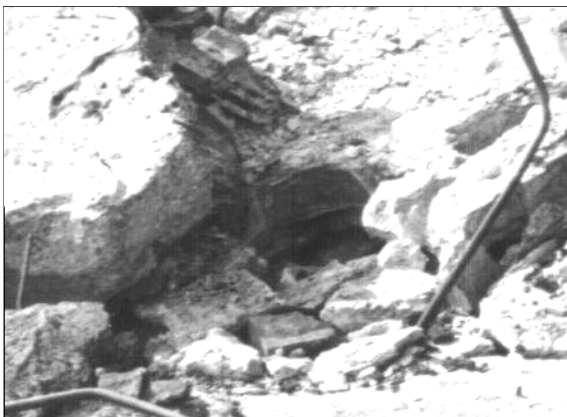
III. 10: Round opening for the pipe of the ventilation through the reinforced concrete roof of morgue 2 of crematorium II in Birkenau. Section enlargement of III. 9. © Carlo Mattogno
