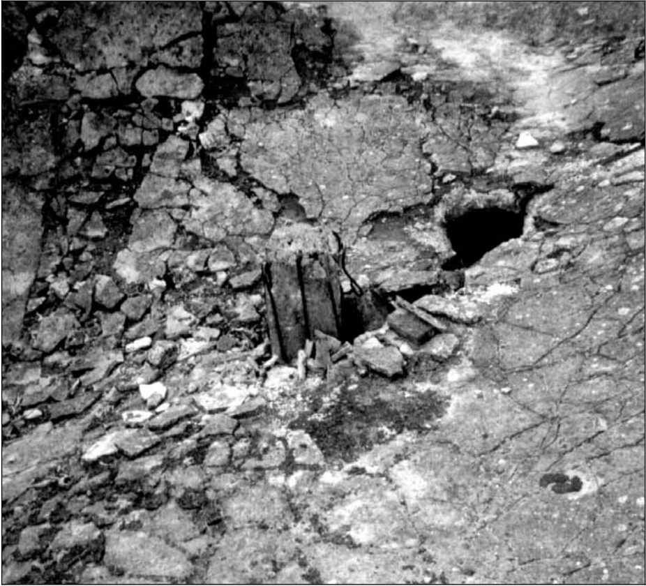
III. 8: Morgue 1 of crematorium II at Birkenau. Concrete pillar protruding from concrete roof slab and the crack produced by the pillar. August 2000. © Carlo Mattogno.
