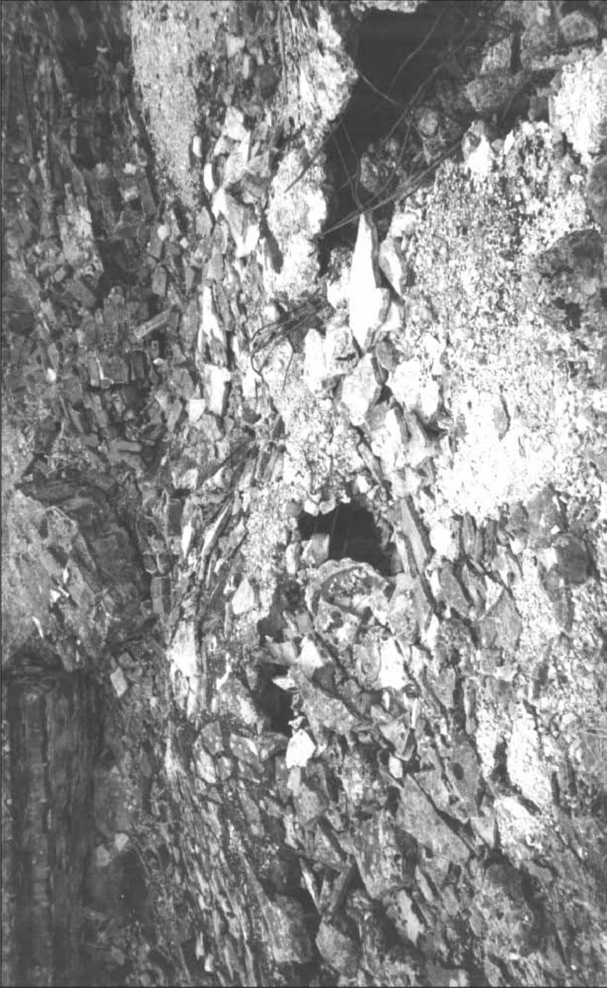
III. 34: Concrete roof of morgue 1 of crematorium II in Birkenau in August 2000. Provan's opening 8 (in the center) and continuation of crack (see photo 33), of which opening 8 is a part. © Carlo Mattogno
