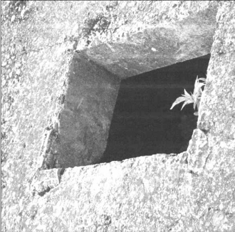
III. 12: Ceiling of the oven room of crematorium III. First ventilation opening (seen from the west). © Carlo Mattogno
