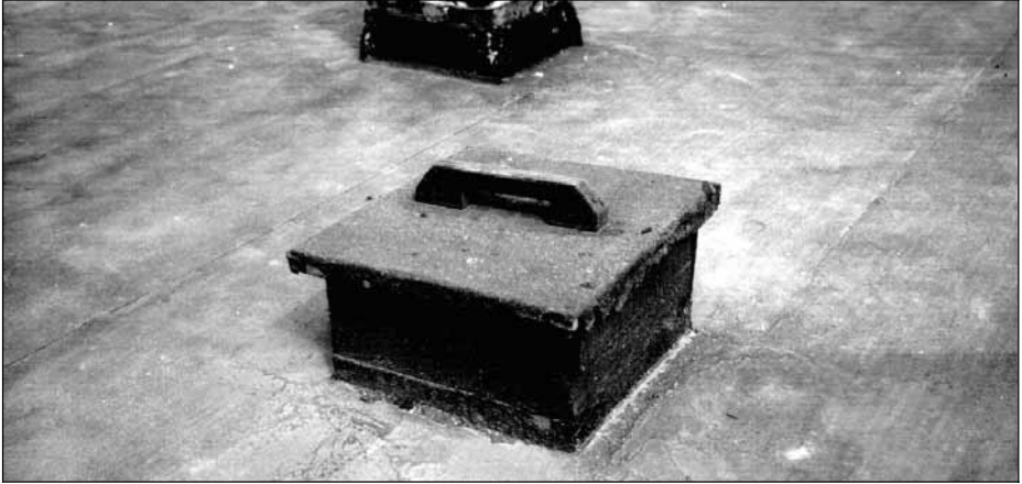
III. 12: Photo of the roof of the morgue. One of the four shafts constructed by the Poles after the war. © Carlo Mattogno.
