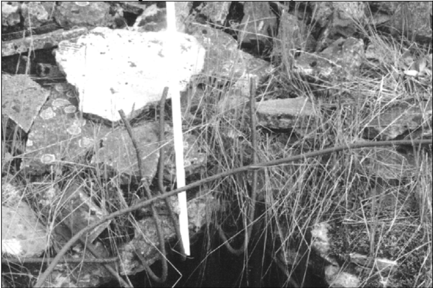
III. 24: Concrete roof of morgue 1 of crematorium II in Birkenau. Reinforcement bars of Provan's opening 7 in June 1990. © Carlo Mattogno
