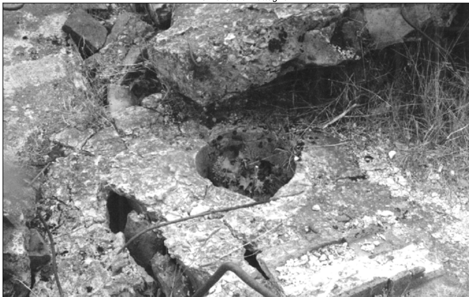
III. 11: Round opening for the pipe of the ventilation through the reinforced concrete roof of morgue 2 of crematorium II in Birkenau. October 1991. © Carlo Mattogno
