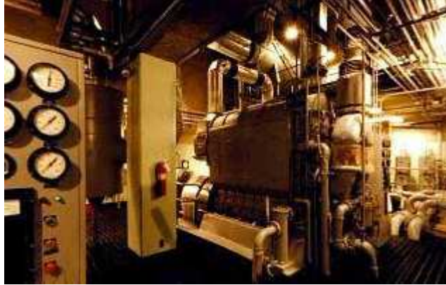
Greenbriar's Power Center
