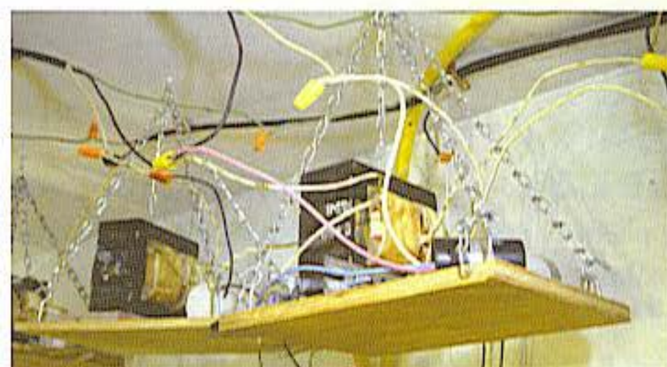
Place ballasts on shelves so that they are up and out of the way.
