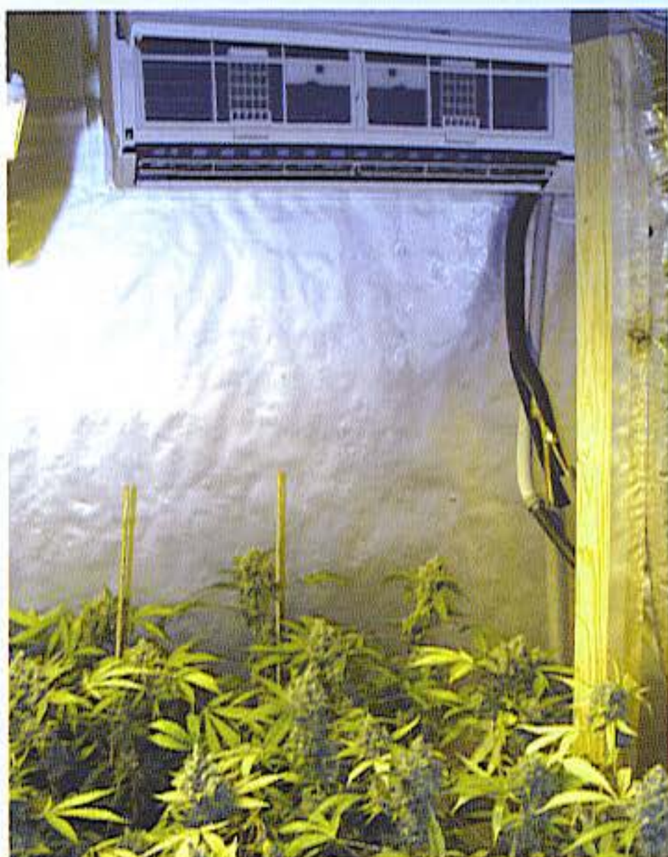
This air conditioner lowers grow room temperature and humidity. The hot radiator is outside, about 10 feet (3 m) away.
