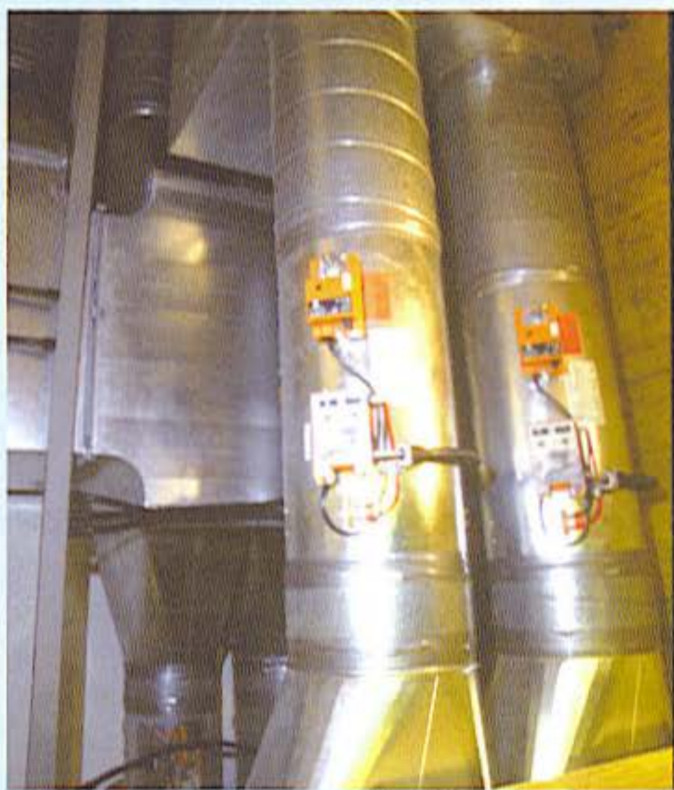
Ozone generators are located inside ducting. Grow room air mixes with ozone in ducting and big metal box. Air smells fresh and clean once treated properly with ozone.
