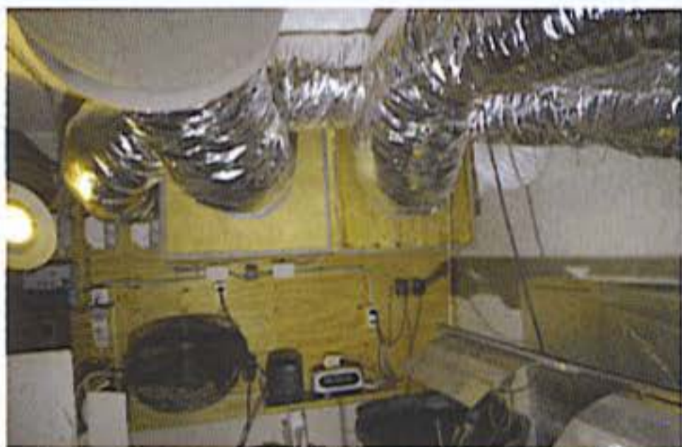
This grower uses insulated ducting to dampen noise and vibrations caused by moving air.
