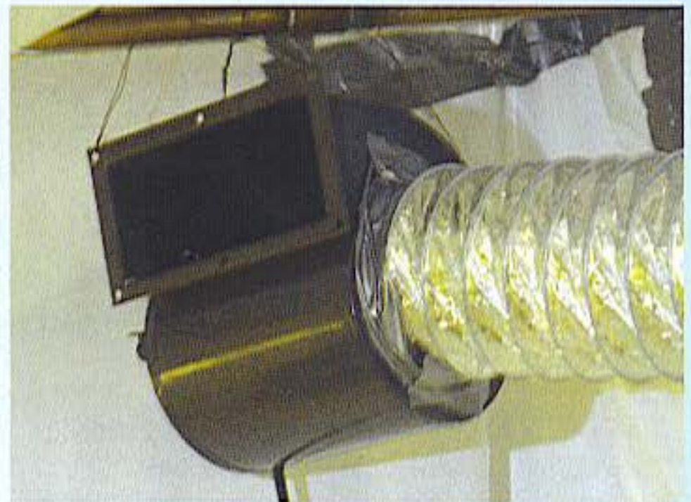
This blower is at the end of intake air ducting. The main fan is at the other end.
