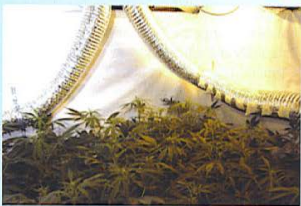
Intake air ducting has holes covered with duct tape. Air flow is directed by removing pieces of tape.
