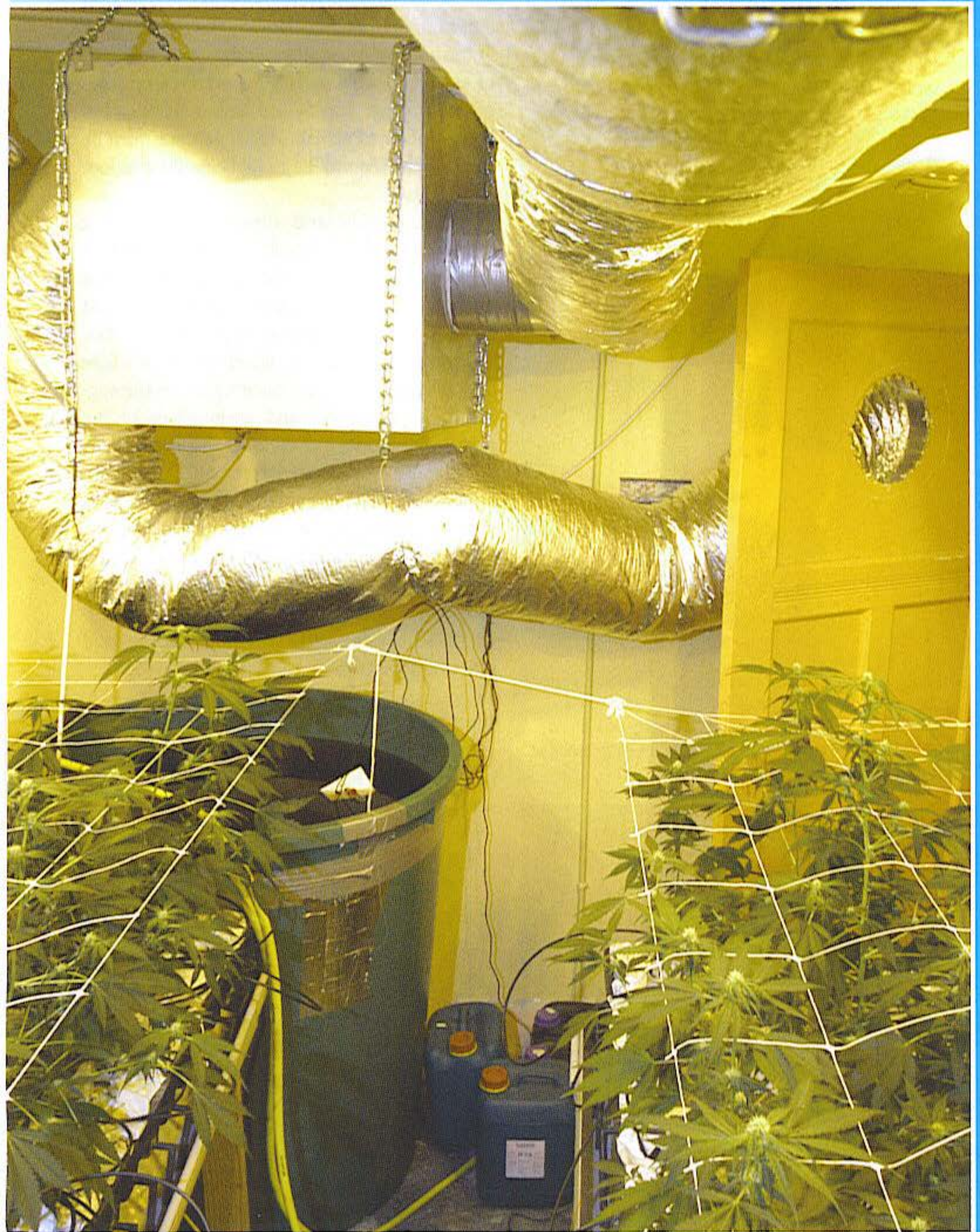
A carbon filter and ozone exchange box dominate the landscape in this Dutch grow room.
