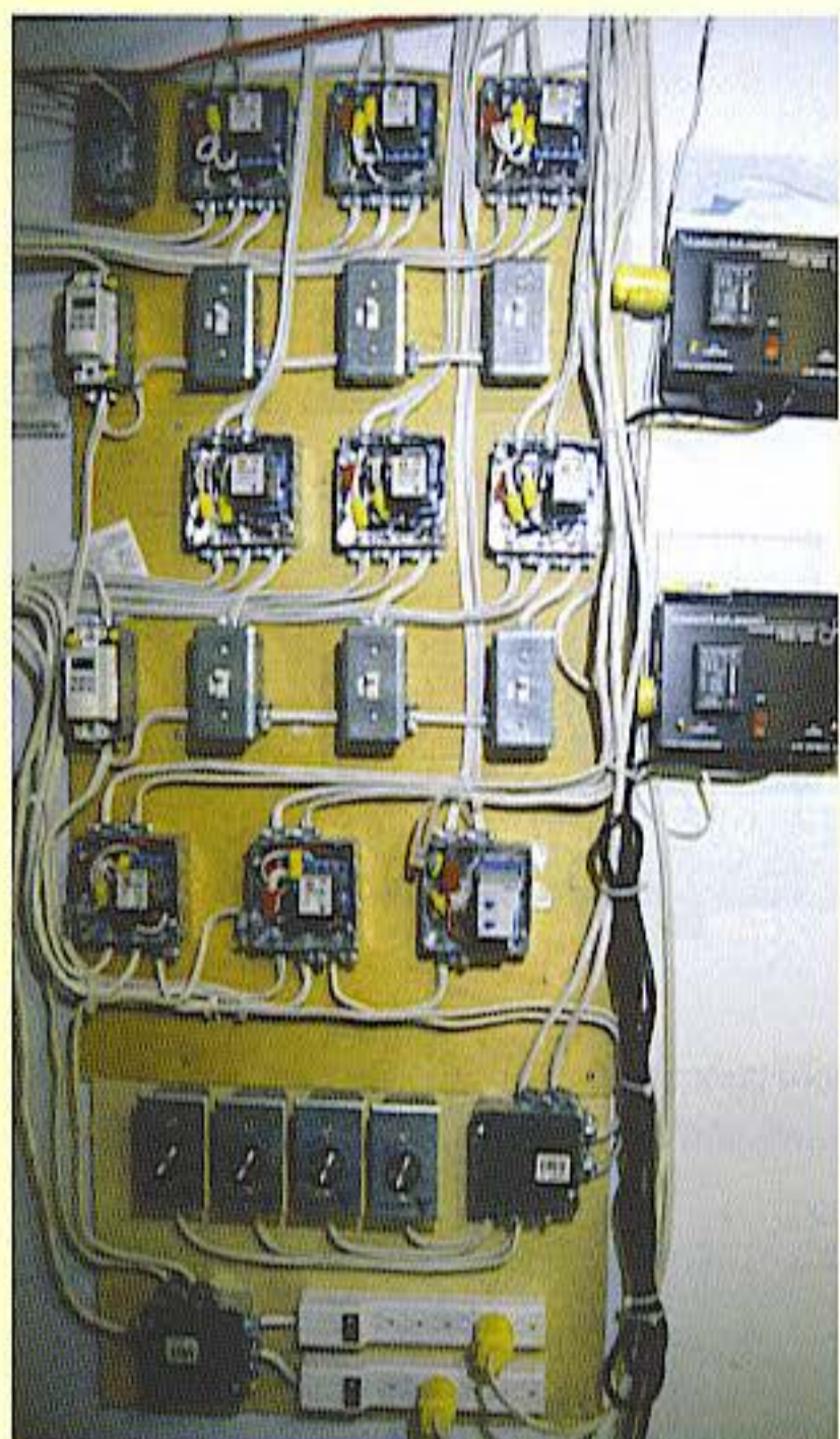
Fixing all wiring and electric devices to a control panel makes control and troubleshooting easy.
