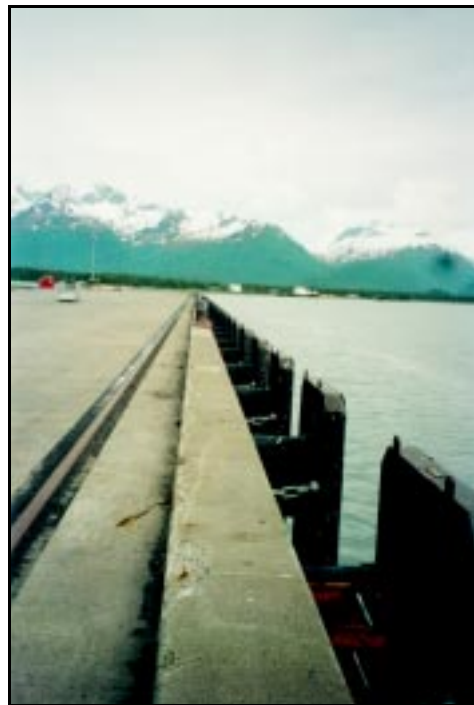
Rubber-Cushion Fendering System at the Port of Valdez
