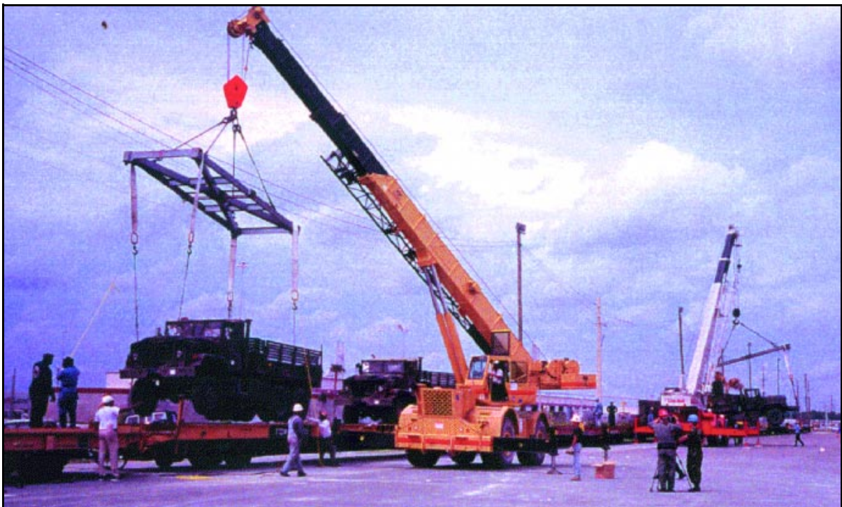
Mobile Cranes at Blount Island
