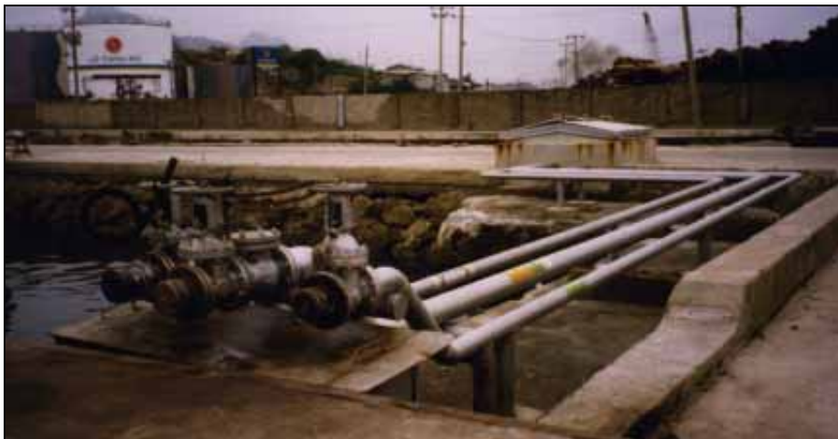
POL Facilities at Port of Mokpo (storage tanks in background)
