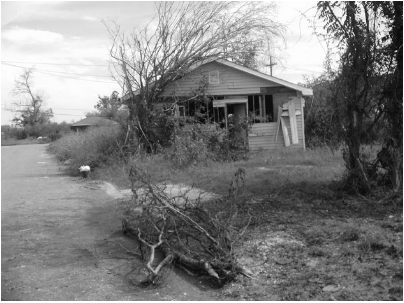
Figure 7.1. A heavily damaged house near Jourdan Road, in the Lower Ninth Ward, October 2006. Photograph by the author.
