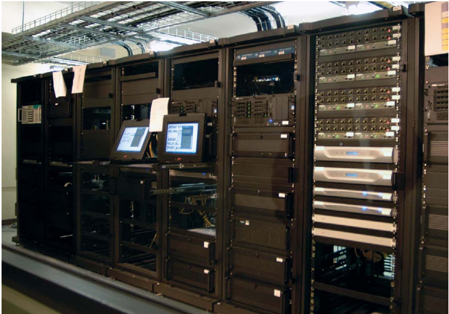
Engineering TOC Entercom Communications Kansas City
