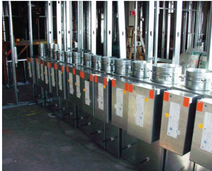
Mechanical VAV Boxes
