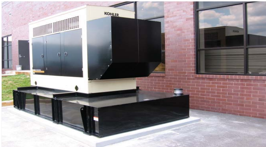
Back Up Generator
