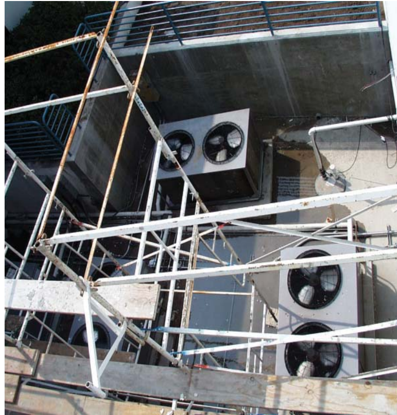
Roof Top Mechanical Equipment
