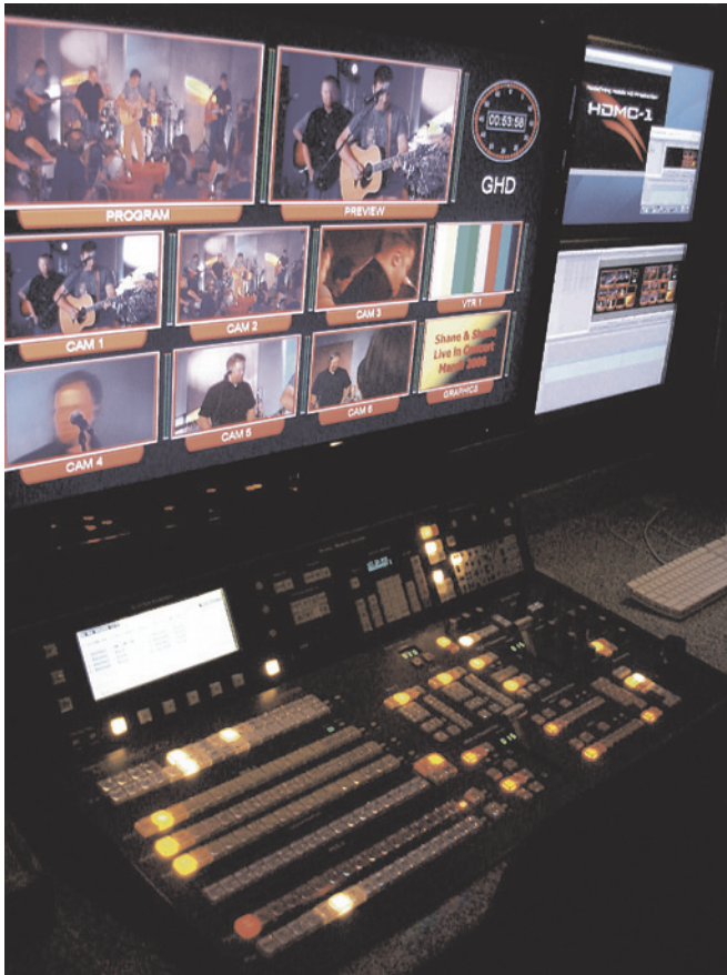
FIGURE 3.15 A small control room.
