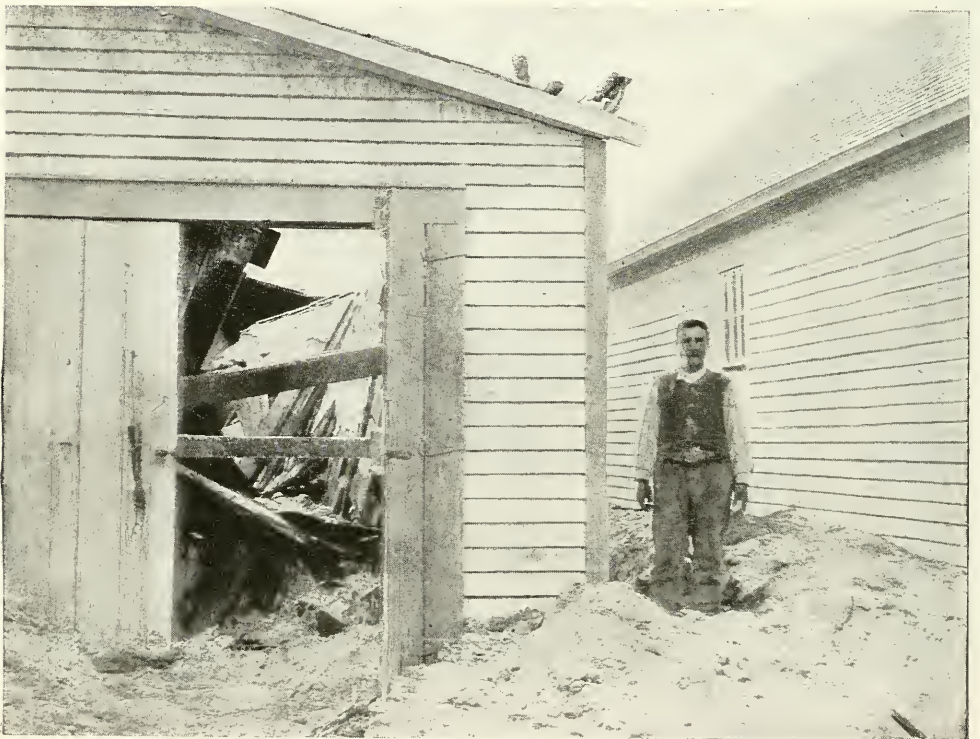
Photo by W. J. Erskine SHOWING ROOF OF FISH HOUSE, AT KADIK BROKEN DOWN FROM WEIGHT OF ASHES. JUNE 14, 1912
