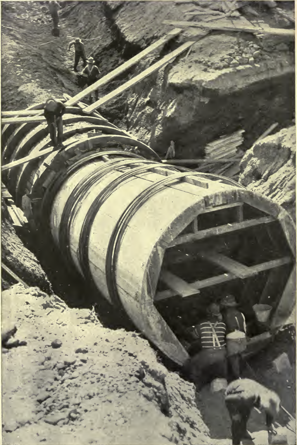
ANOTHER VIEW OF AN INVERTED SIPHON: IT IS BUILT OF CONCRETE HEAVILY REINFORCED WITH STEEL (SEE PAGE 576)
