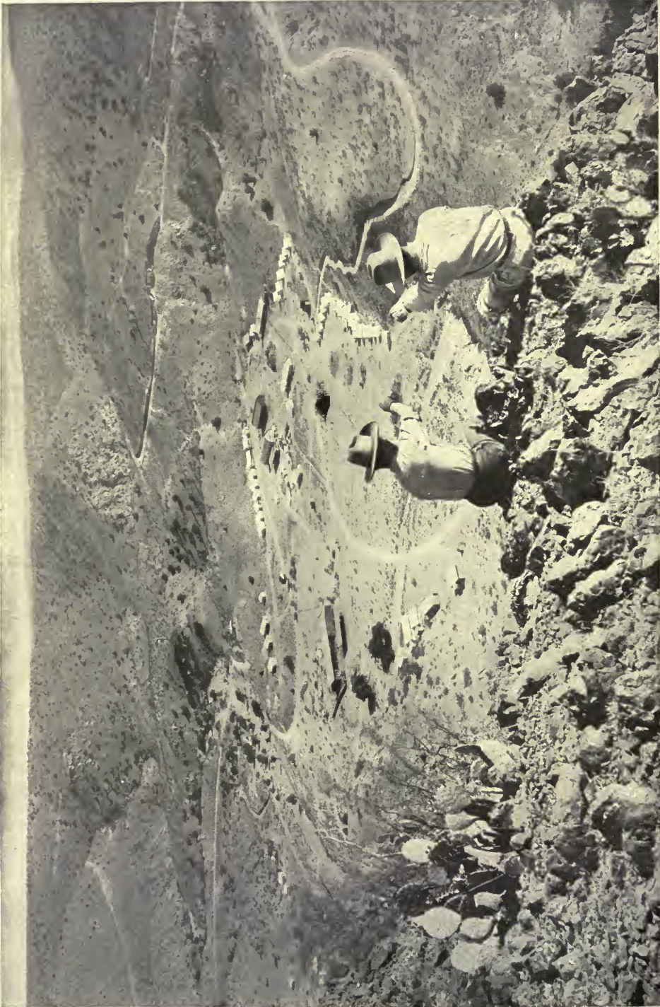
BEGINNING OF THE GREATEST PROJECT OF THE RECLAMATION SERVICE: THE NEW CAMP AT ENGLE DAM SITE, RIO GRANDE VALLEY, NEW MEXICO
