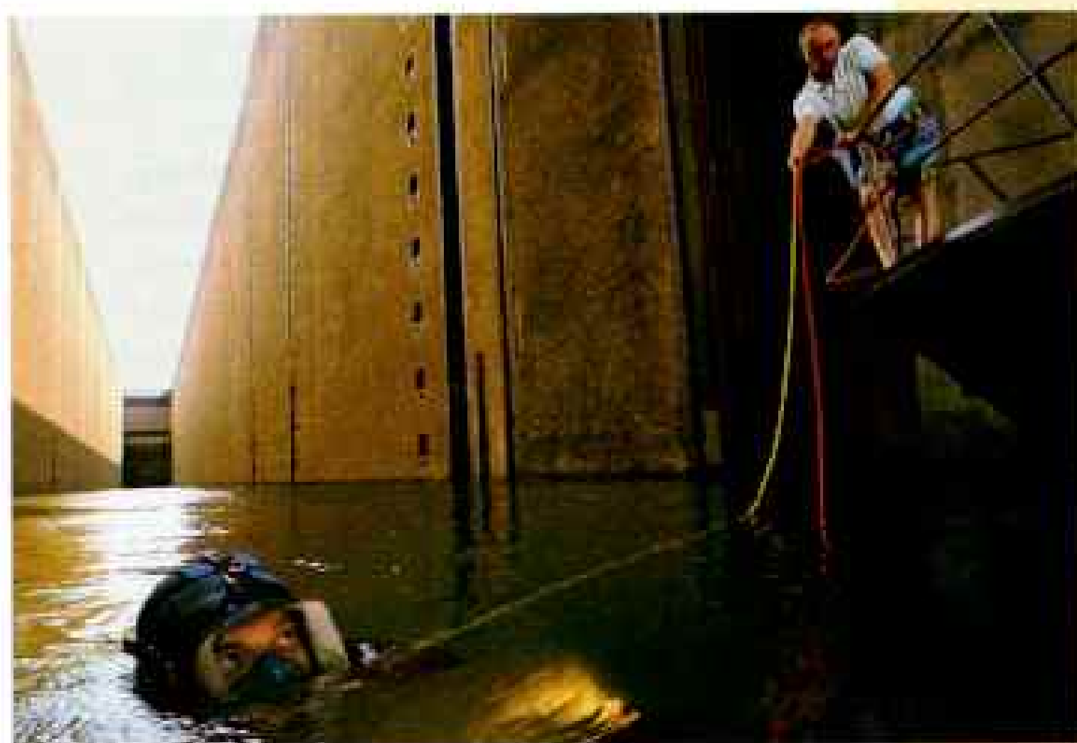
A diver with a video camera checks for cracks in Leerstetten lock, which raises ships seven stories to the next lock level.
