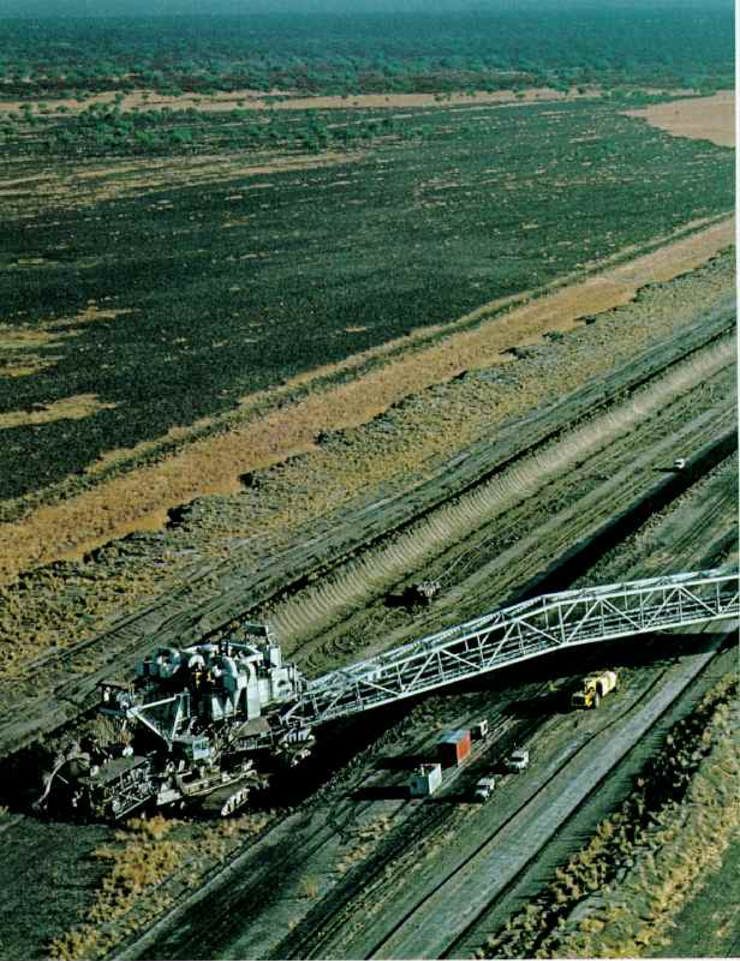
Mighty swath cut by a gargantuan earthmover will become the 360-kilometer-long Jonglei Canal. Funded jointly by Sudan and Egypt, the canal will divert part of the White Nile from its present course through the Sudd, where much of the water is
