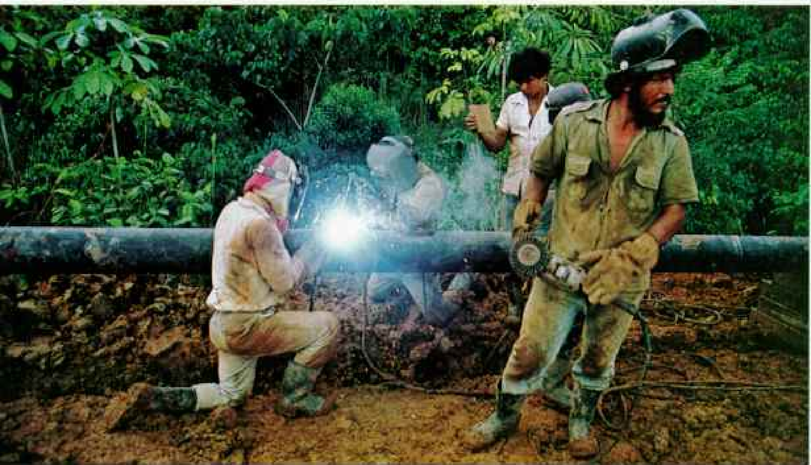
Gamble becomes boom: Welding fuses a pipeline near Andoas, after a 1978 oil strike helped boost Peru's known reserves by almost 20 percent. When the state first struck jungle oil in 1971, it urged foreign companies to join the probe. All failed except U. S.-owned Occidental Petroleum, which persevered, making strikes that allowed Peru to export a billion dollars' worth of oil last year.
