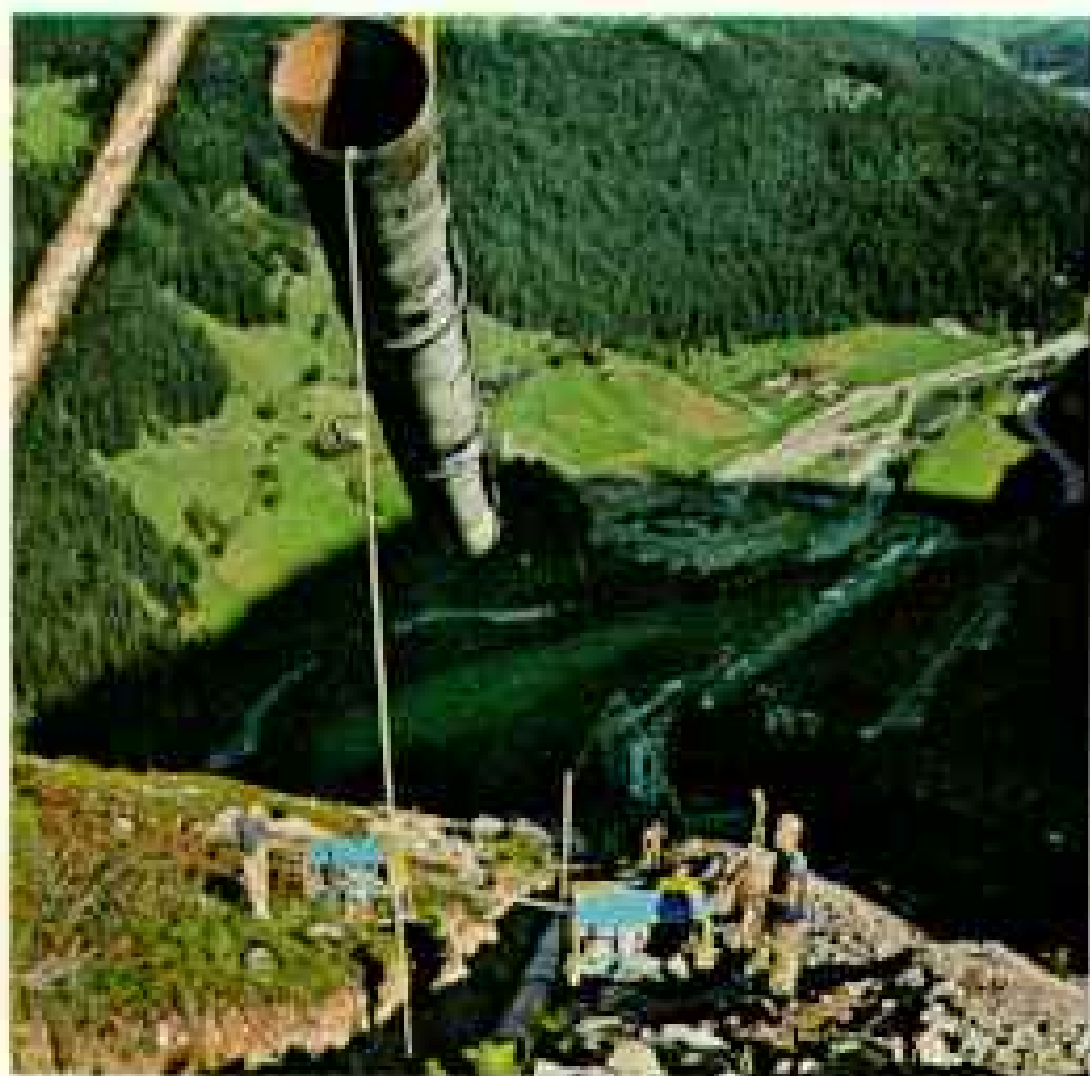
In rocky terrain, the pipe is laid on a cushion of sand to protect it from jagged projections.
