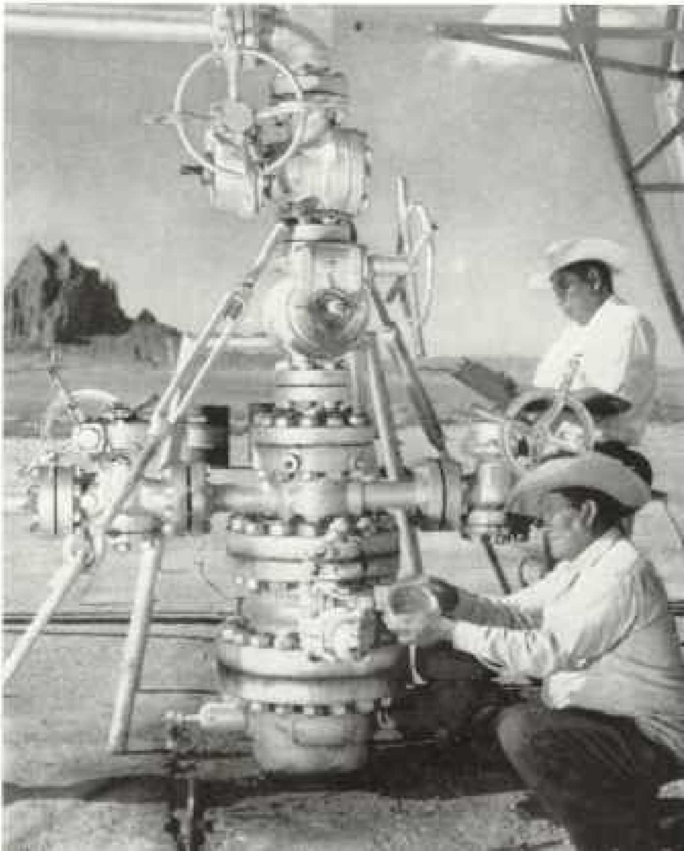
Maze of valves regulates the flow of a helium-bearing natural gas well. These Navajos check wellhead pressure below Ship Rock, a butte in New Mexico.
