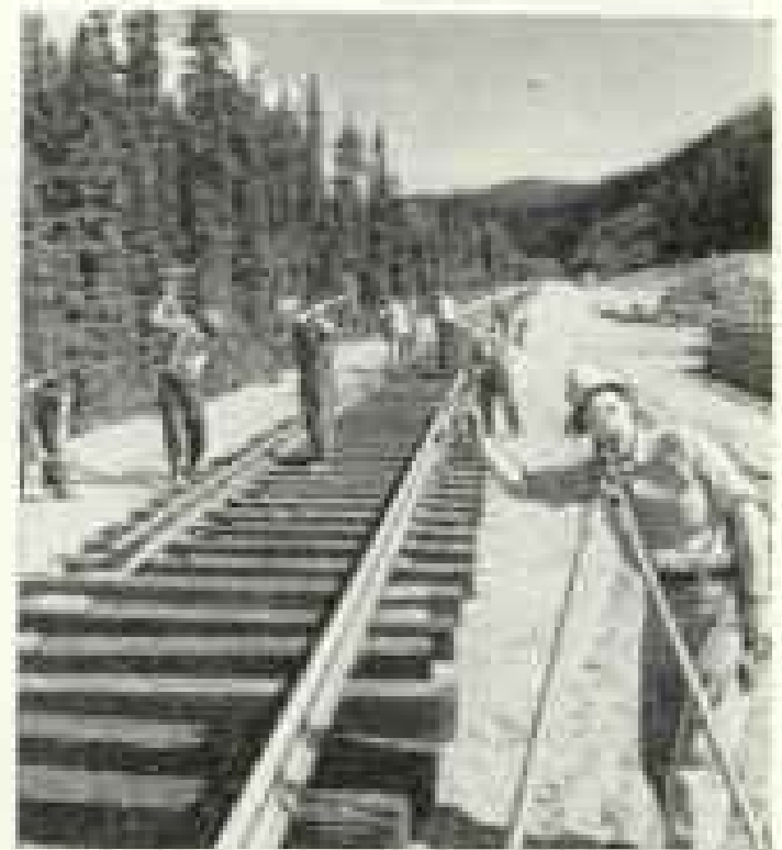
New, heavier rails and tie plates are spiked to chemically treated ties. Maintenance crews give daily attention to roadbed.
