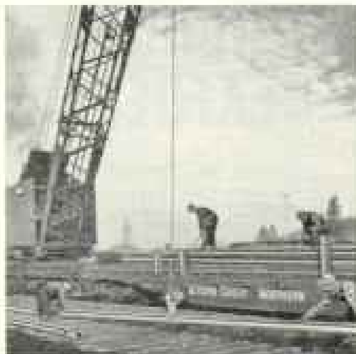
Steel rails are lifted by crane from G.N. flatcars and placed in position.
