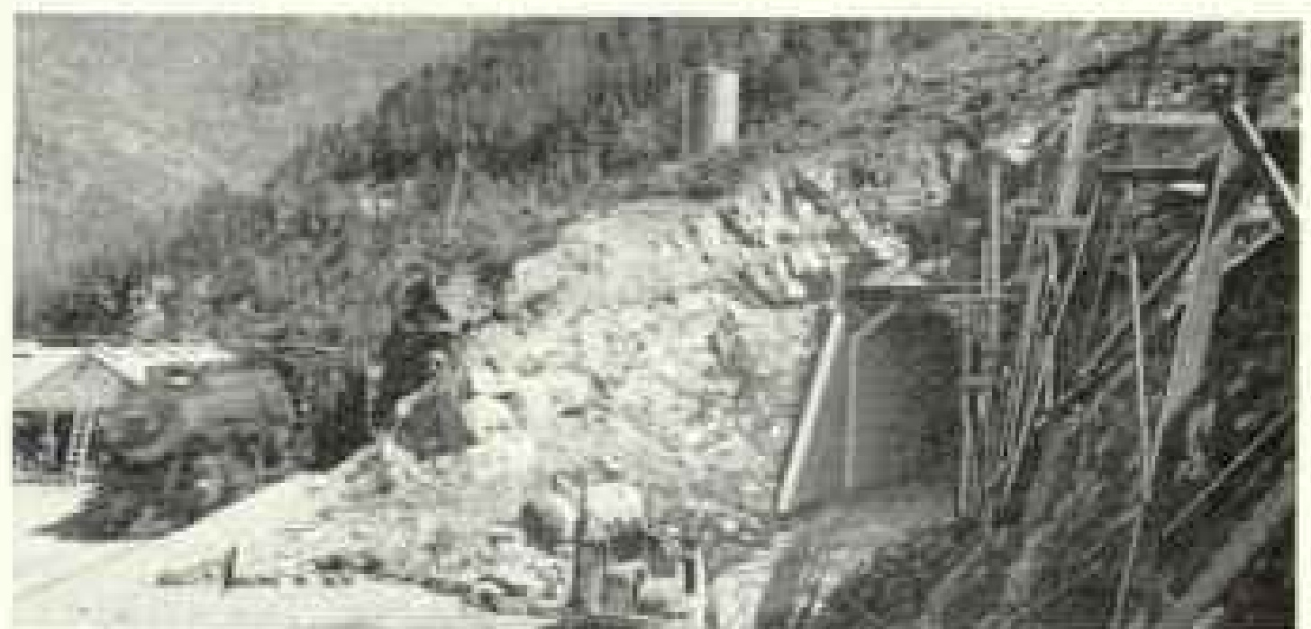
West portal of one of three new tunnels through solid rock on G.N. main line in the Montana Rockies to expedite train movements.
