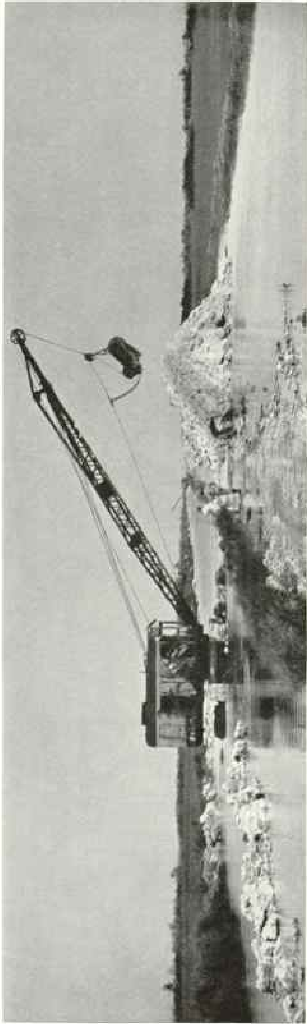
TO BUILD THE TAMiami TRAIL, THE ROADBED (RIGHT) WAS CLEARED OF MUD AND THEN FILLED WITH ROCK BLASTED FROM A PARALLEL DITCH
