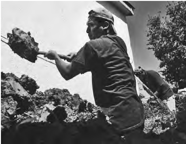
Rebuilding New Orleans, 2006. Following Hurricane Katrina, large numbers of undocumented workers, such as this laborer from Mexico, came to the region and performed much of the clean-up work. MARIO TAMA/GETTY IMAGES.
