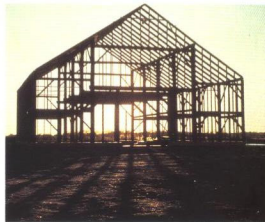
Above: The clarity of the spatial hierarchy of the original barn frame both informed and resolved the parti.
