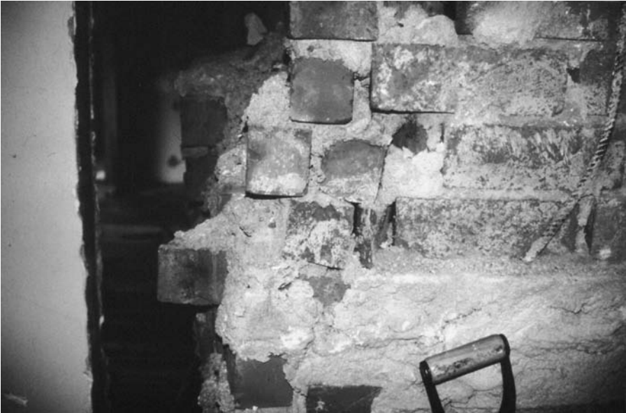
Figure 8.10 One of the numerous poorly built fireplaces damaged by the Northridge earthquake.
