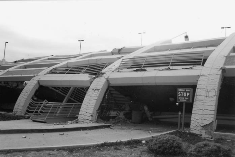
Figure 1.1 Parking structure that collapsed during the 1994 Northridge earthquake, California State University, Northridge Campus.
