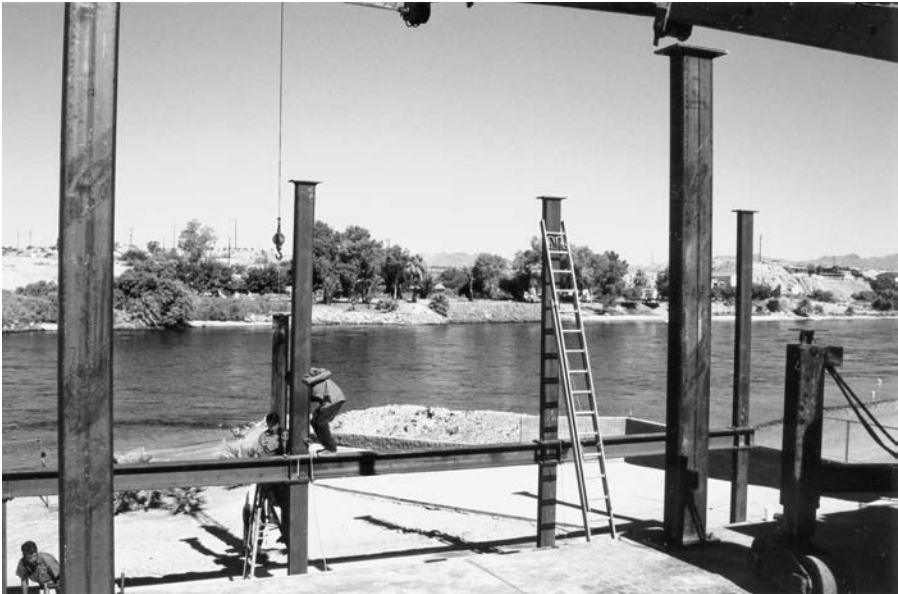
Figure 8.13 First stages of erection of the steel frames that will provide additional support against wind and seismic forces to the type-V building.
