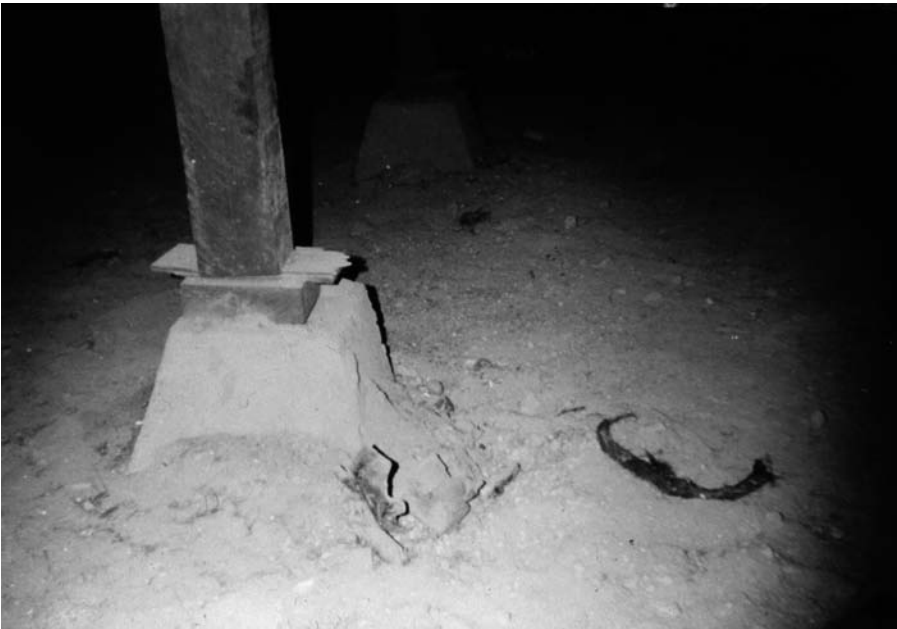
Figure 8.3 Rough-and-ready workmanship. Wood wedges inserted under the support assembly.
