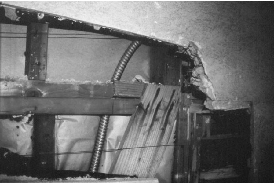
Figure 8.7 Cripple wall damaged during the Northridge earthquake.
