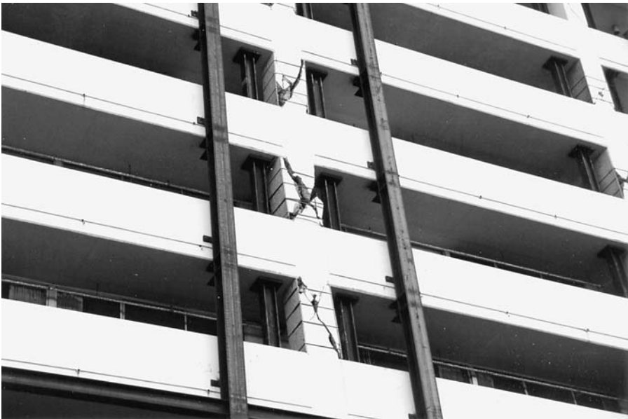
Figure 1.9 Reinforced-concrete columns severely damaged in the Northridge earthquake, Champagne Towers, Santa Monica, CA.
