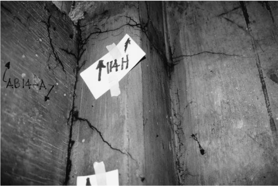
Figure 3.9 Earthquake-caused cracks in cast-in-place concrete beams.
