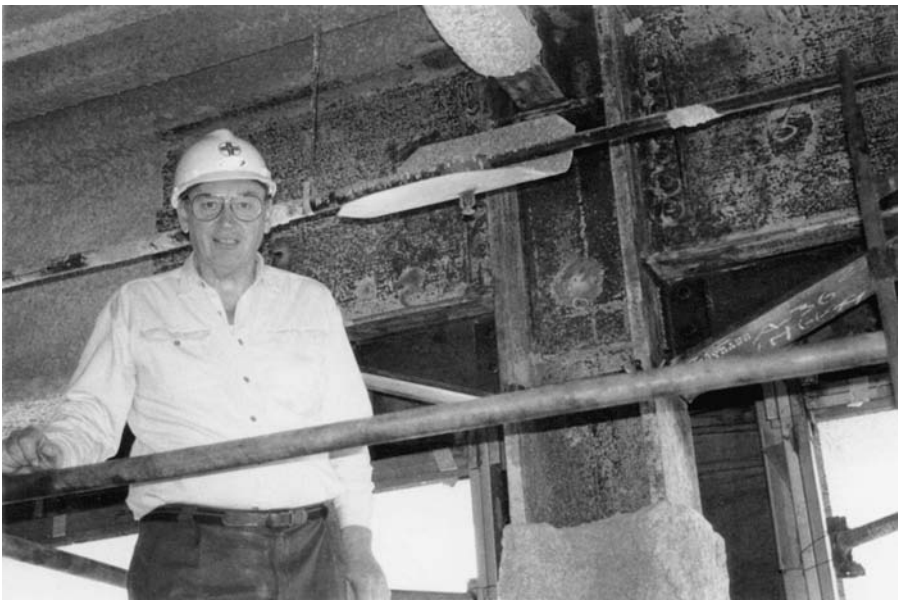
Figure 12.8 Above: Column web fracture within the connection panel zone in the subject structure during the Northridge earthquake. Below: The author during inspection of one of the first retrofittings of cracked welded steel moment-frame structure connections following the 1994 Northridge earthquake.
