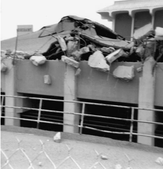
Figure 1.3 Detail of parking structure that collapsed during the Whittier Narrows earthquake of 1987.
