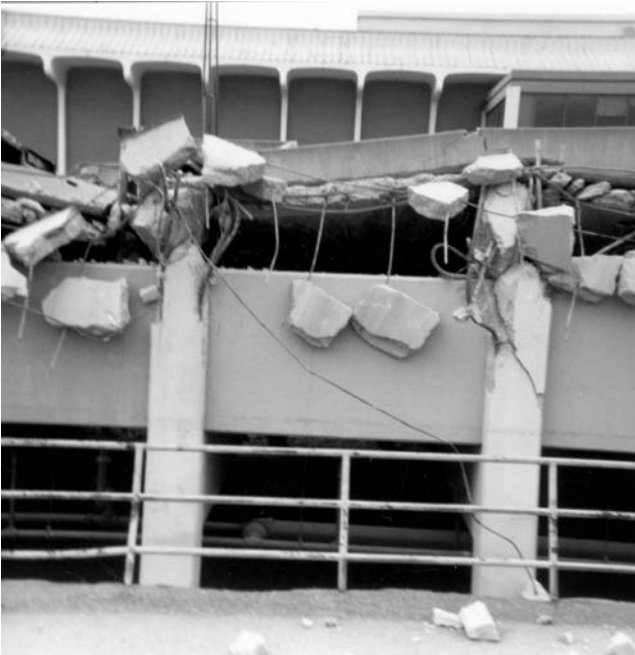
Figure 1.19 Exterior columns that supported the second floor broke at the second-floor beam–column intersection, fashion center parking structure.
