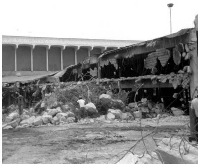
Figure 1.20 Collapsed upper floor and a large portion of the collapsed parking structure, later demolished, Whittier Narrows earthquake, 1987.
