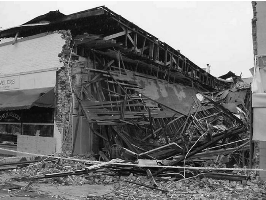
Figure 7.1 Unreinforced masonry buildings do not fare well in earthquakes. The photo shows the collapsed “House of Bread” in the city of Paso Robles, California during the 6.5-magnitude San Simeon earthquake of December 2003. The Old Clock Tower, symbol of Paso Robles, built in 1892 in the corner of the same building was also destroyed when the second story of the structure collapsed onto the street during the earthquake. (Courtesy of the University of California Berkeley Library. Photo: Janise E. Rodgers.)
