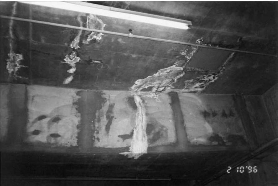
Figure 3.10 Water damage in roof structure due to seepage from the plaza above.
