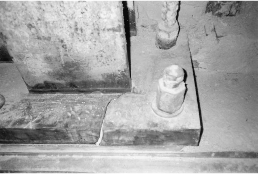
Figure 1.16 Cracks in 4-in.-thick base plates during the Northridge earthquake, Oviatt Library Annex Building.
