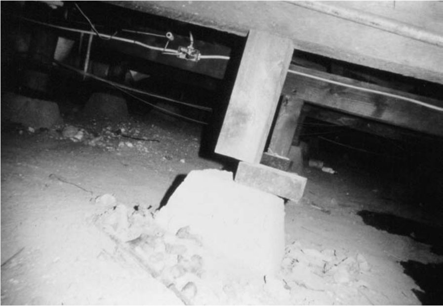
Figure 8.2 Dangerously unstable support to the floor above.
