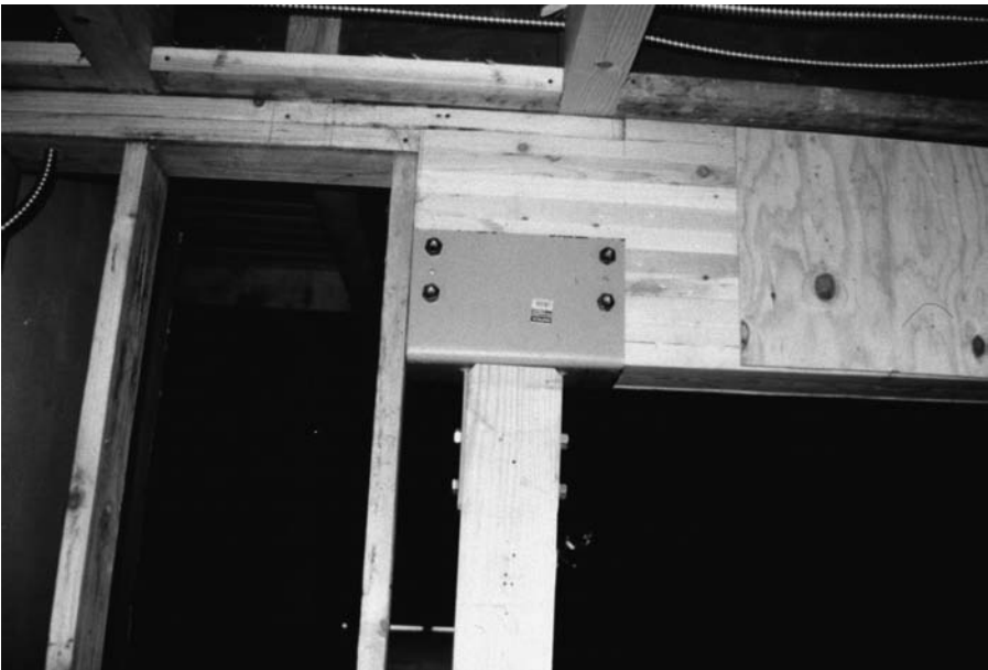
Figure 8.5 Properly engineered metal connector used to join individual wood elements in the retrofitting of an earthquake-damaged residential building.
