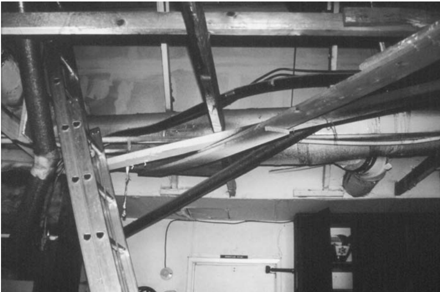
Figure 8.8 Common sight in earthquake-damaged garages coupled with poor workmanship.
