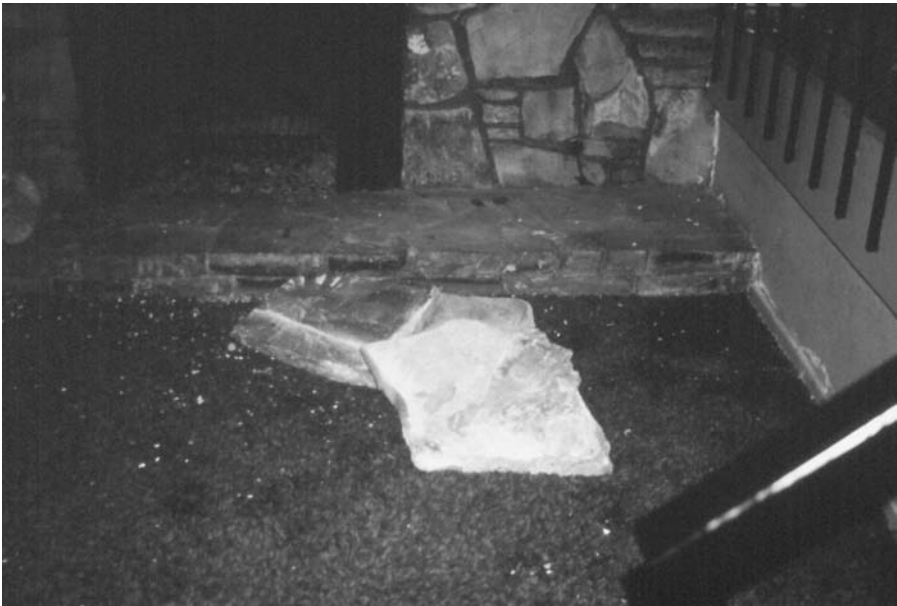
Figure 8.9 Two-story stone fireplace that collapsed during the Northridge earthquake.
