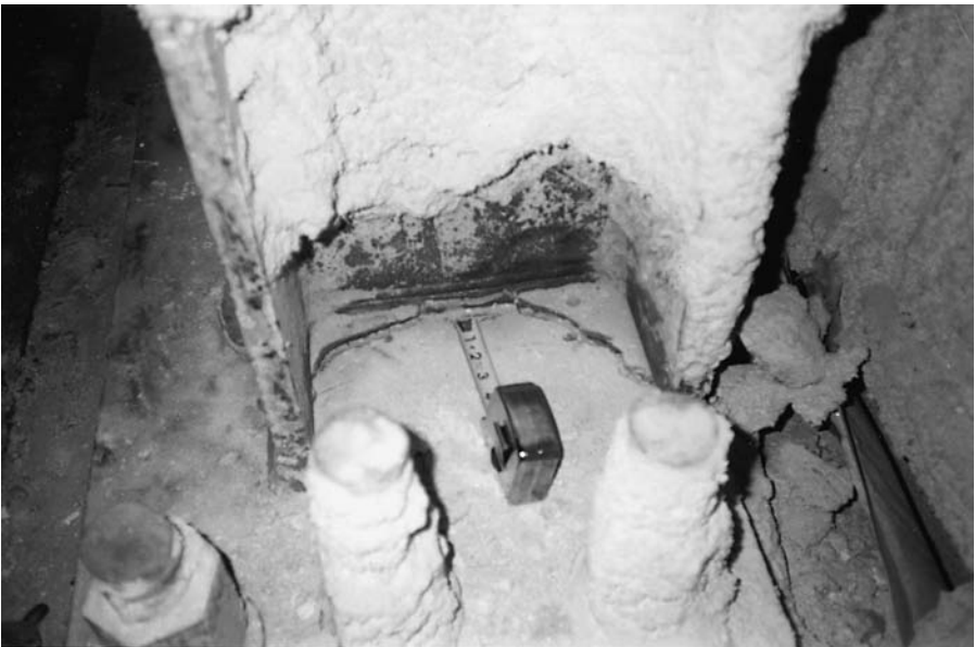
Figure 1.17 Shear failure at perimeter of frame leg–base plate solidly welded connection, Oviatt Library Annex Building. Note the crack in the center and the initial stage of shear failure on the left.
