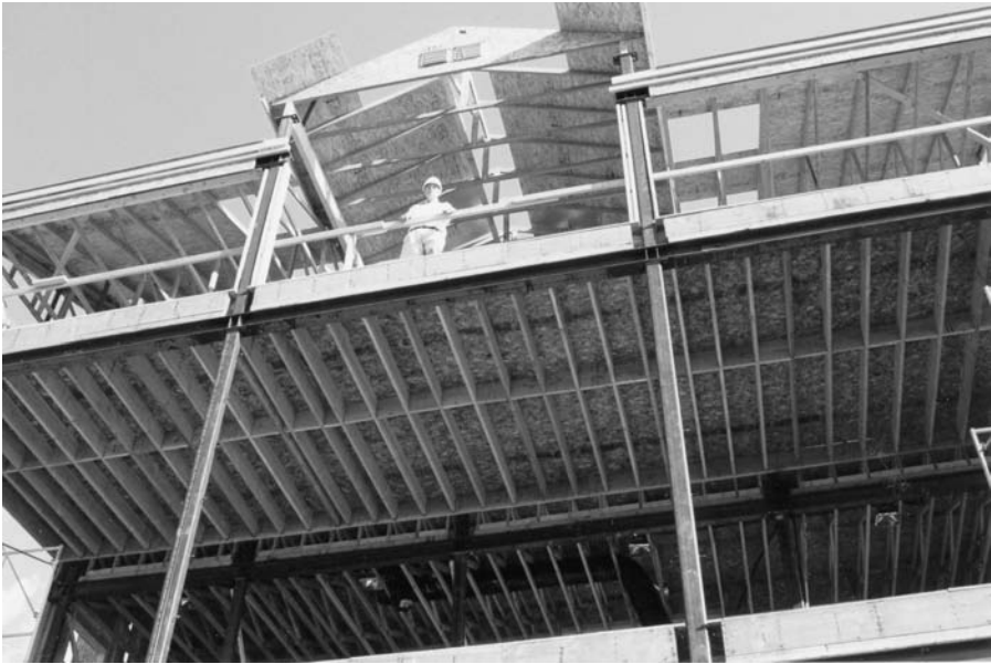
Figure 8.14 View of the second and third floors of the north elevation with the steel frame in place.
