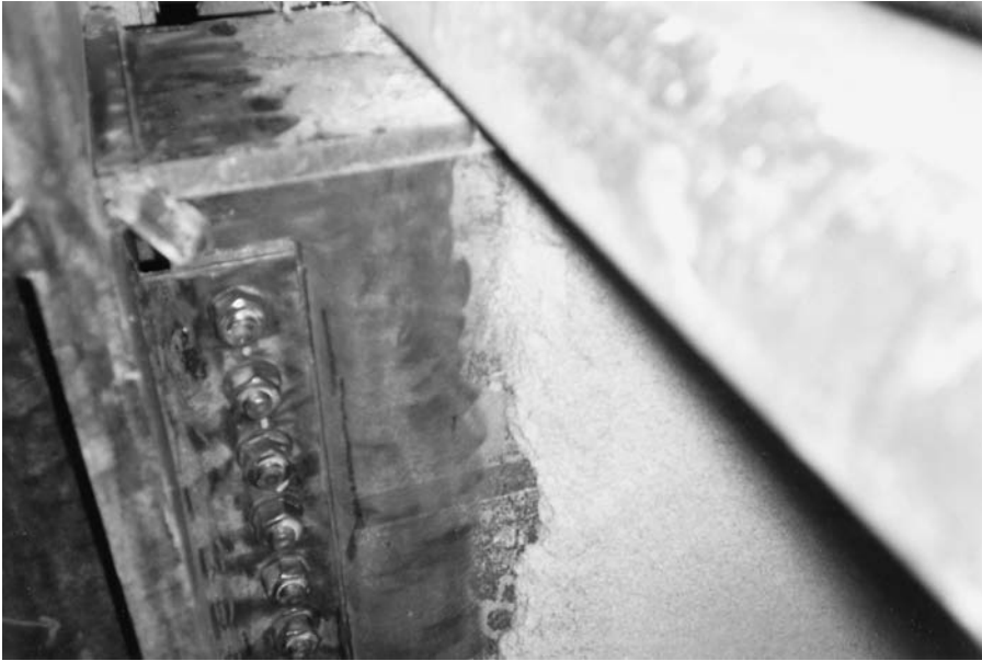
Figure 1.15 Left: crack in beam web during the Northridge earthquake, Anthony Building, Department of Water and Power, Los Angeles County.
