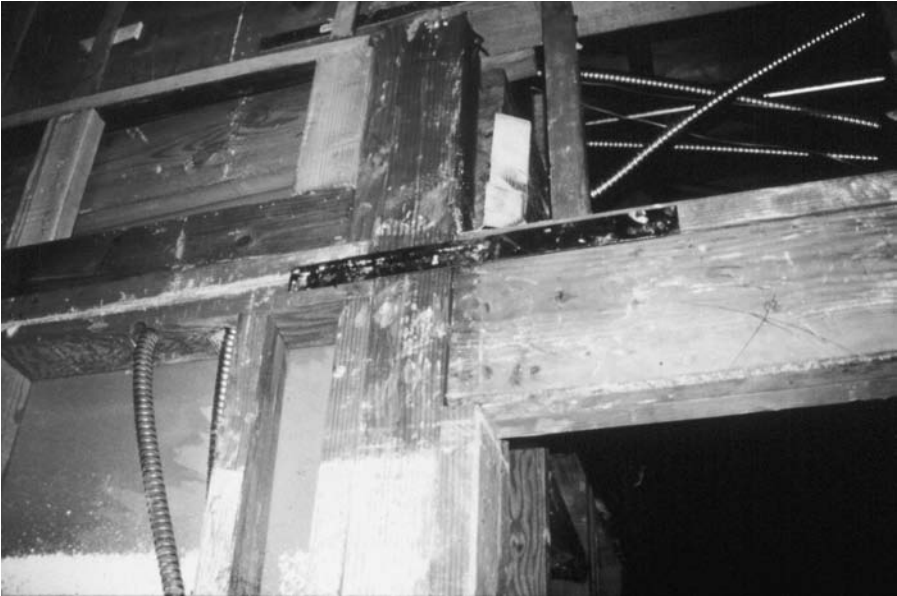
Figure 8.4 Inspection of damaged buildings found plumber straps in lieu of engineered metal connectors to join individual wood elements.
