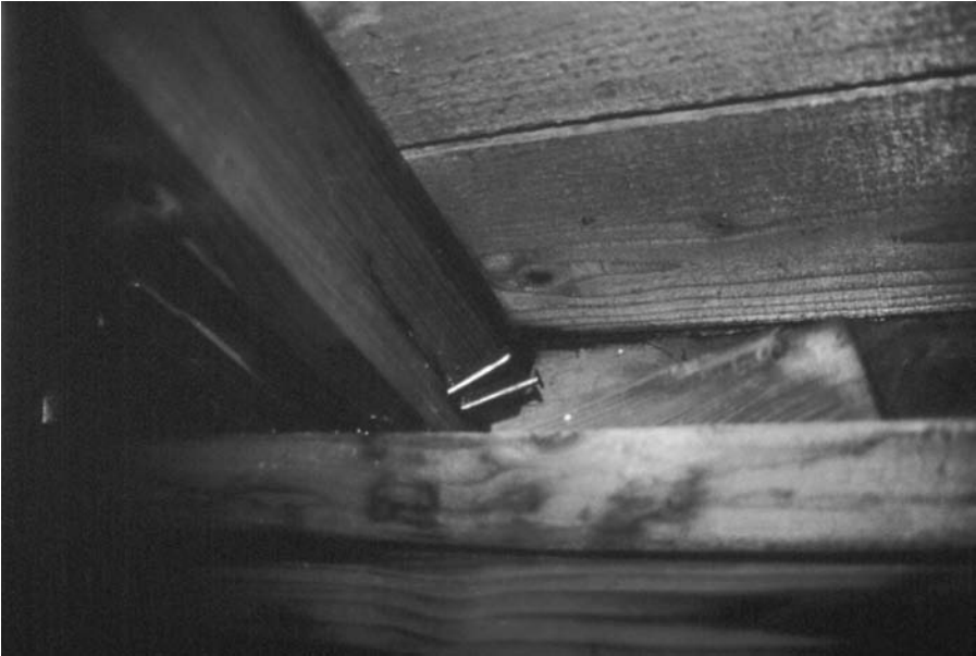
Figure 8.6 Toenailing, an unsafe practice to face a violent earthquake, which pulled out the nails.
