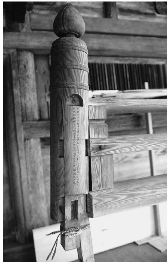
Figure 9.39 Detail of a former repair of the Buddhist temple of Cyōjū-ji. The date and signature of the repair have been inscribed inside the new element
