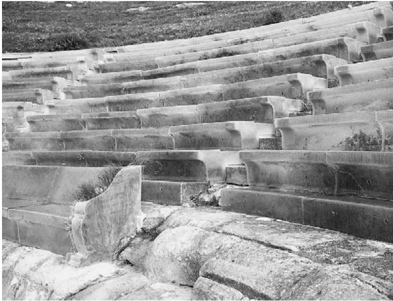
Figure 10.2 The antique theatre of Eraclea Minoa in Sicily was restored in the 1960s, using transparent plastic display as a 'scientifically' planned protection. The microclimate under the plastic, however, has seriously threatened the preservation of the original stones. In 1996, the authorities decided to remove the plastic, and design a more appropriate form of protection
