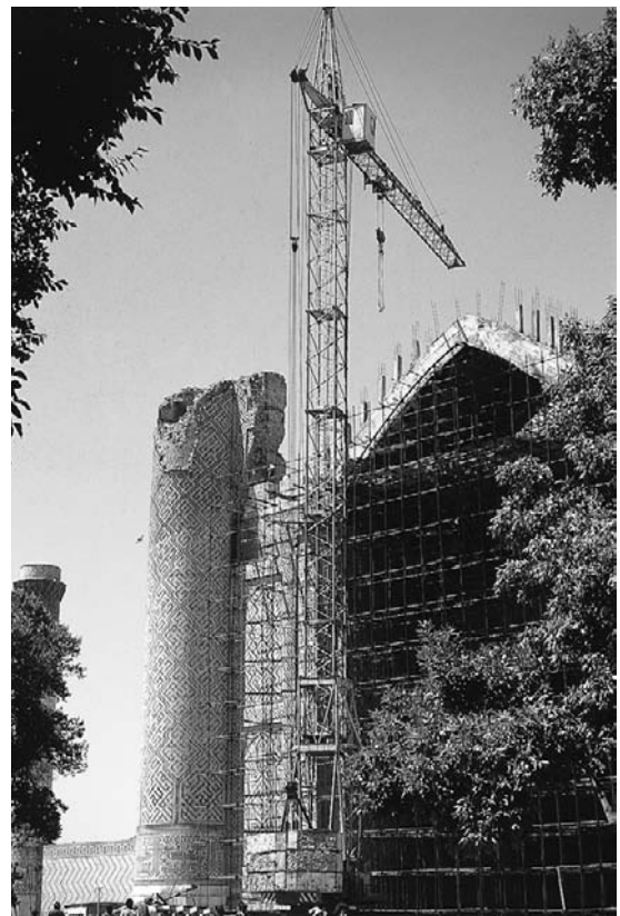
Figure 10.8 Reconstruction of Bibi Khanum mosque in Samarkand, in 1997, using reinforced concrete for the structure and traditionally produced bricks and tiles for the surface. New glaze differs from the old in quality and for its slightly lighter tonality
