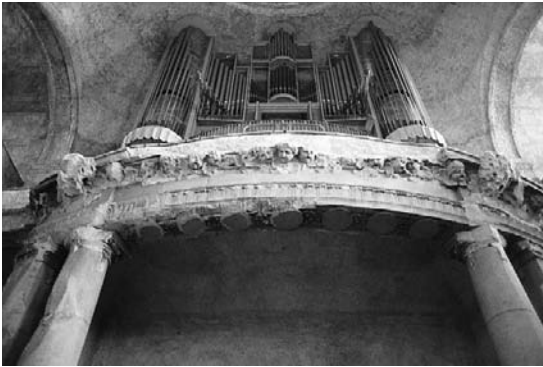
Figure 9.13 The restoration of war-damaged Kreuzkirche in the centre of Dresden is an example of minimum intervention; instead of reconstruction, rough cement was applied on damaged surfaces – providing also good acoustics
