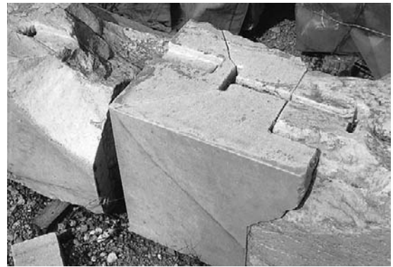
Figure 7.8 A detail of ancient marble restored by Balanos showing the cut in original material for the insertion of new stone and an iron cramp
