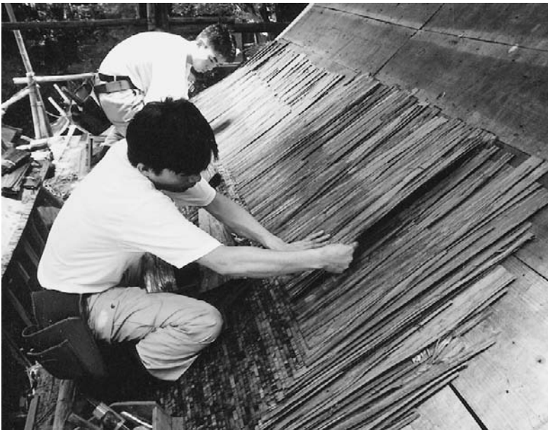
Figure 9.37 The roof of the Kasuga Shrine being rebuilt during recent restoration (c. 1994). (Kasuga Shrine management)
