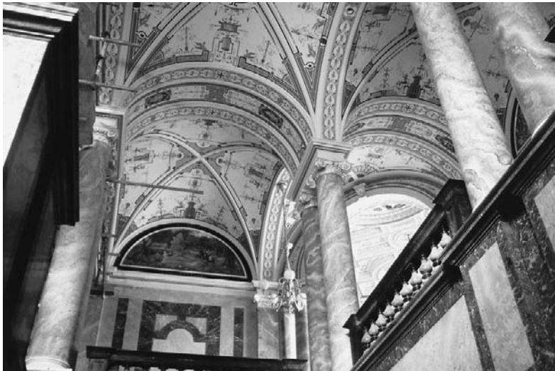
Figure 9.12 The Semper Opera of Dresden was rebuilt in the 1980s. The foyer area is an example of reconstruction with full colour scheme based of careful archival and field research, as was the case in several restoration projects in the former German Democratic Republic
