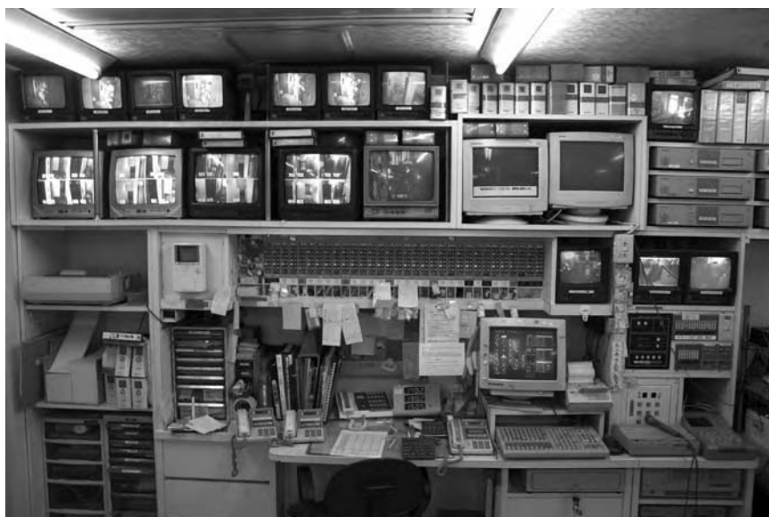
Figure 5.1 Control room, Hotel Maria Teresia, Nanba, Osaka (photo courtesy of Ed Jacob).
