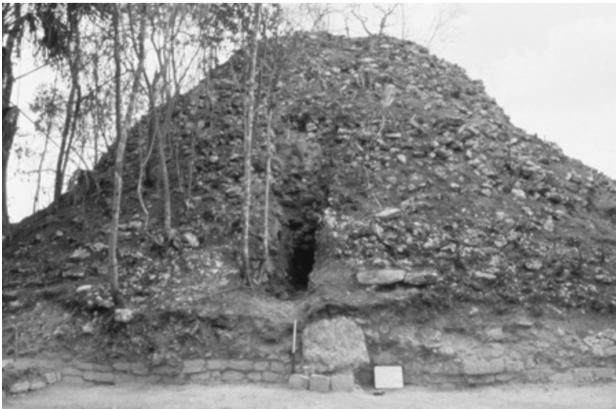
Figure 9.1 Looters' trench in one of the buildings of Plaza Yaxná in Kohunlich. The building was trenched on all four sides; the looters were not successful but damaged the building to a point where its restoration became practically impossible
