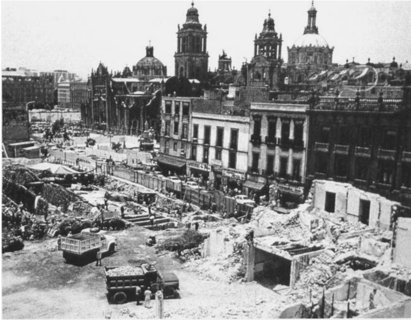
Several modern buildings were demolished in 1980 in order to excavate the area where the House of Eagles was discovered. The Great Temple is to the left in the picture.
