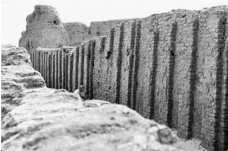
FIGURE 7.4 The mudbrick wall of the Early Dynastic Shunet al-Zebib (the funerary enclosure of King Khasekhemwy) at Abydos, Egypt.
