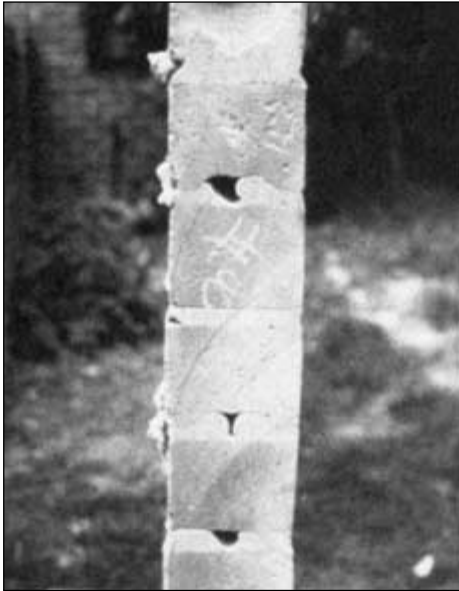
FIGURE 6.2 Incompletely Filled Bed Joints (The Magazine for Masonry Construction, May 1990).
