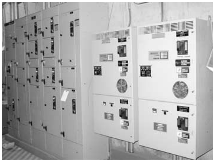
FIGURE 9.13 Motor control center (cabinet on left) and variable frequency drives (two boxes on right).
